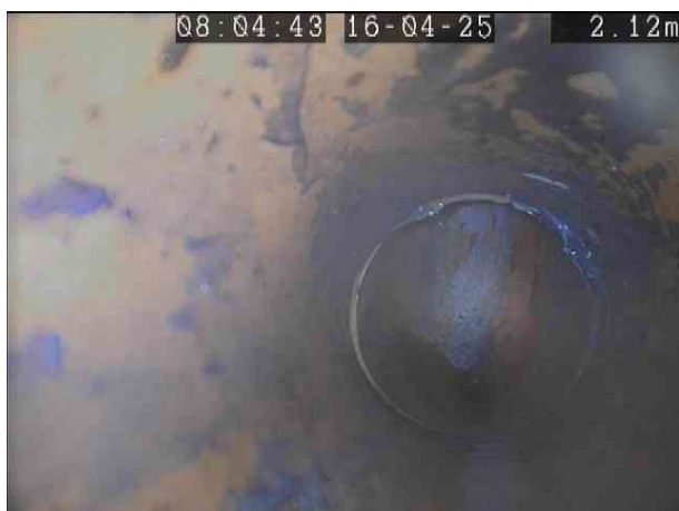
SVP3X_3c829e4c-8699-4725-abf1-1212e879c6a6_20250422_204411_315.jpg, 00:00:22, 2.12 m Pipe material changes to polyvinyl chloride at this point
