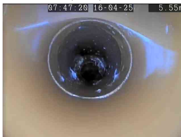
SVP2X_65399523-1535-45ca-9879-d7d9fa23af80_20250422_202449_658.jpg, 00:00:41, 5.55 m Junction at 12 o'clock, 100mm dia
