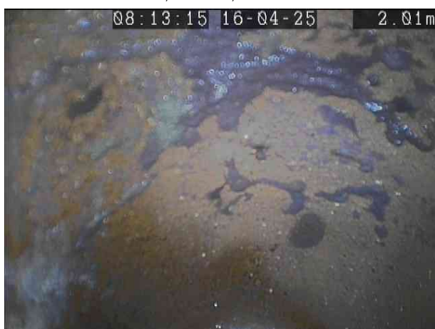
WG2X_44a7ada1-d353-4657-a115-3cef9722ddf6_20250422_205141_535.jpg, 00:00:22, 2.00 m Finish node, gully, reference: WG2
