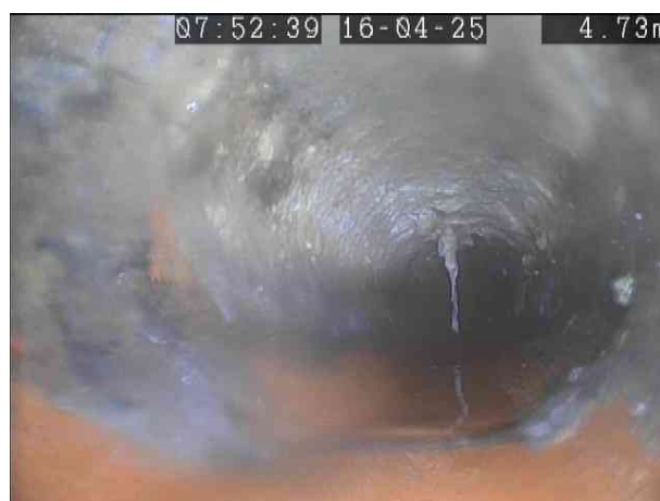
IC1X_e8610c84-1073-4ada-9506-a02aa1d10ae5_20250422_203904_779.jpg, 00:01:39, 4.77 m Survey abandoned, Unable to push any further
