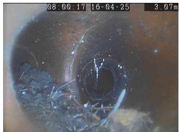
DISUSEDX_cf9fbd5c-465f-42d0-9002-a93d179469b7_20250422_204125_106.jpg, 00:00:38, 3.31 m Junction at 9 o'clock, 100mm dia
