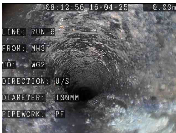
WG2X_2641b69a-66d1-4ee4-a122-f692a65fc24d_20250422_205113_673.jpg, 00:00:00, 0.00 m Start node, manhole, reference: MH3
