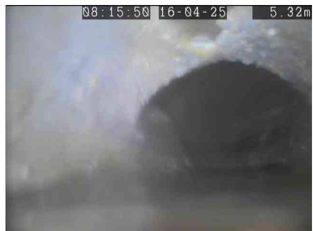
MH3X_e89d4b18-d2d8-426b-8f30-43cd22dc57d6_20250422_205900_637.jpg, 00:00:45, 5.32 m General remark, MH4
