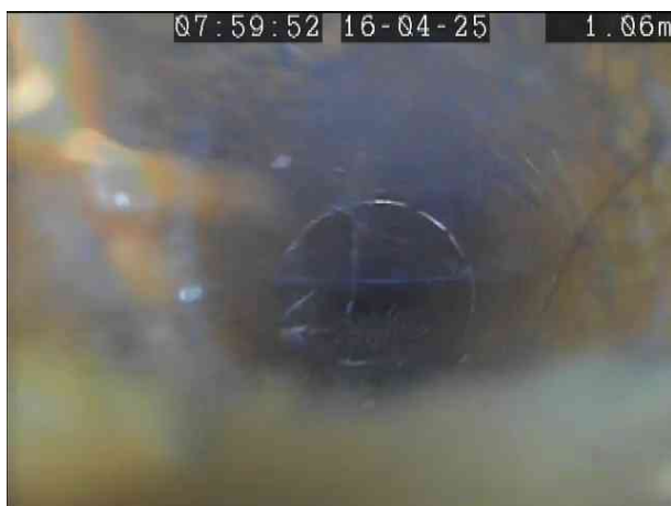
DISUSEDX_043b217d-e816-4ba7-9350-1d089e2ba2b4_20250422_204151_700.jpg, 00:00:13, 1.06 m Roots, mass, 15% cross-sectional area loss
