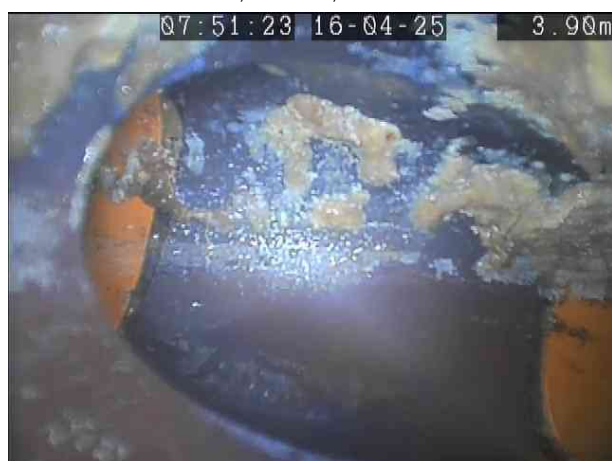
IC1X_acb02c9f-2e38-4489-9f50-ba81d72da4f9_20250422_203712_327.jpg, 00:00:07, 3.90 m Connection other than junction at 3 o'clock, 100mm dia
