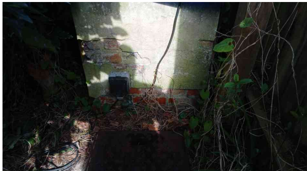
pump chamber with outside socket
