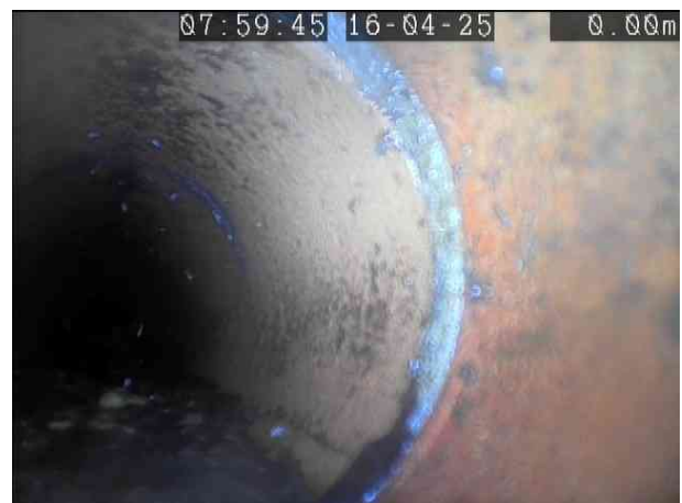
DISUSEDX_d9921927-0f1e-4ee1-8422-190217e6844d_20250422_204046_931.jpg, 00:00:07, 0.00 m Water level, 5% of the vertical dimension
