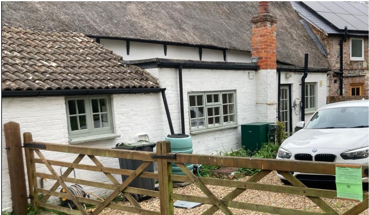
EV charger installed by back door (applicant's photo)
