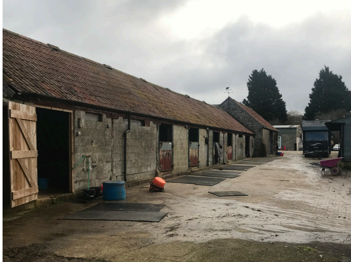
Fig 1 South elevation middle stable section frontage- concrete hardstand to be removed and replace with permeable driveway.
