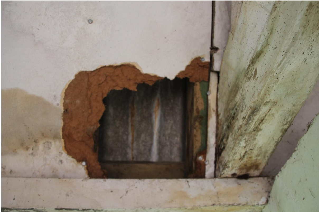
Photograph 3: showing gap in a ceiling panel within central garage area
