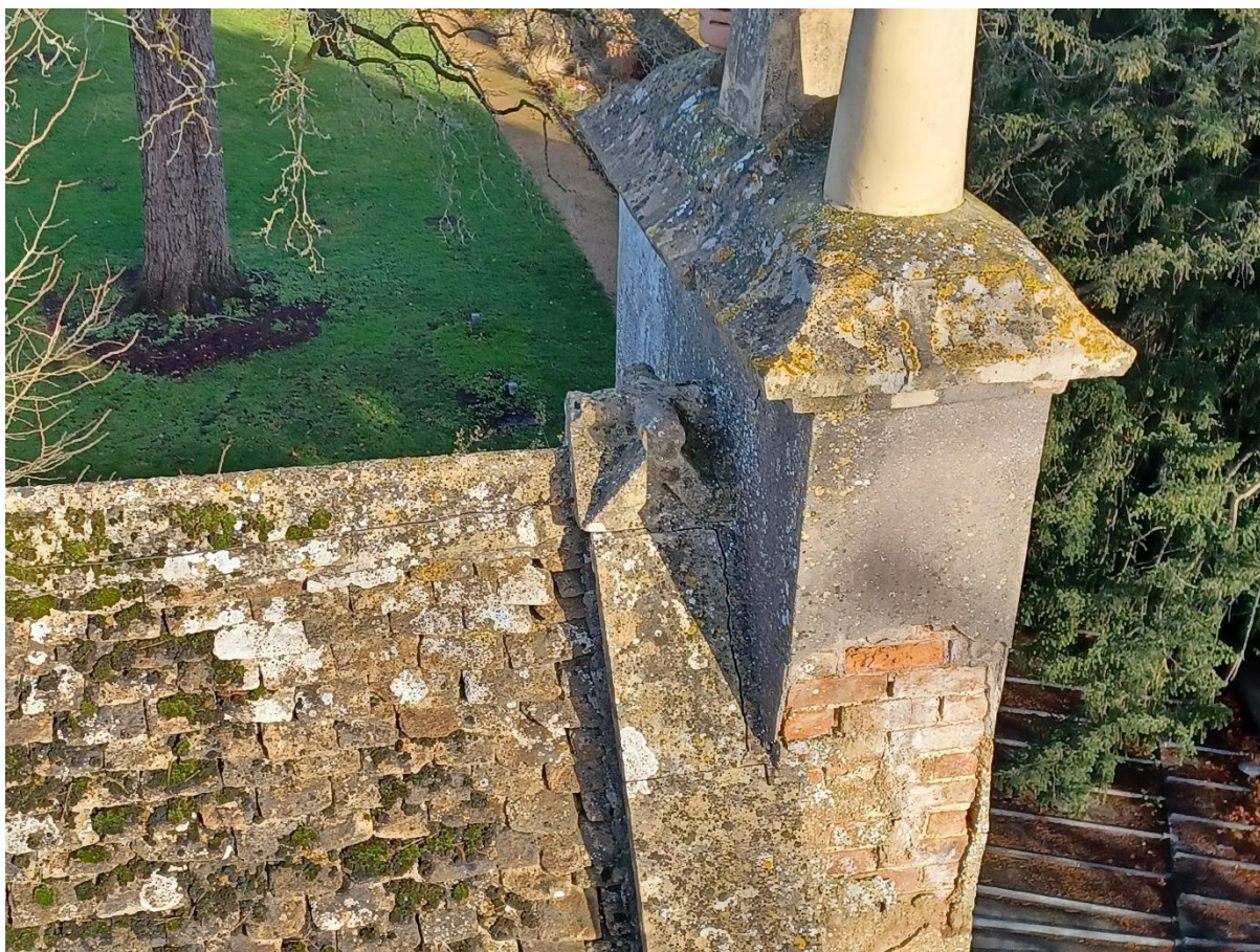
Image 3: showing cementitious render and damage/loss of render, before removal
