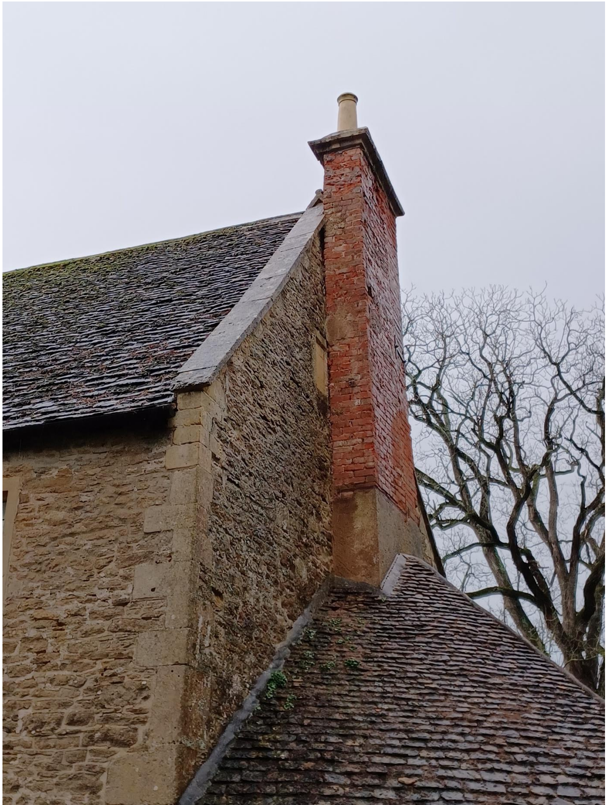
Image 4: showing gap between stack and gable wall
