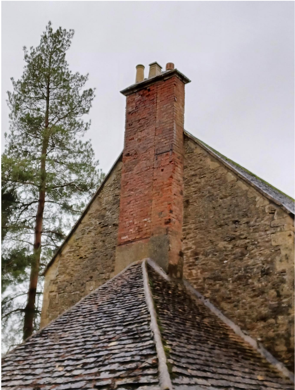
Image 2: Overview of chimney once the render was removed, showing two distinct chimney stacks and damage to brickwork
