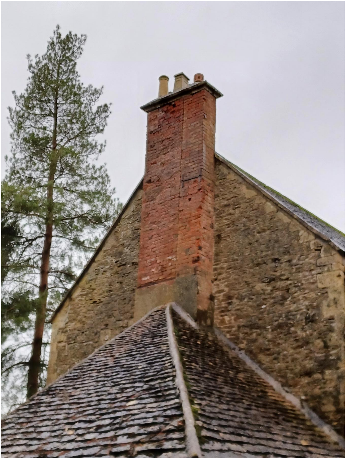
Image 1: Overview of chimney with the render removed, showing two distinct chimney stacks and damage to brickwork
