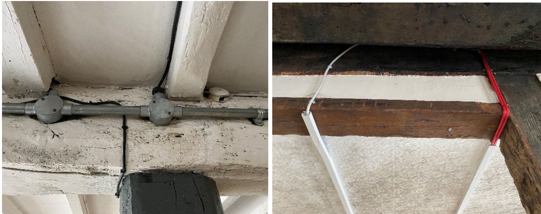
Figure 25: surface mounted wiring avoids impact to timber frame, but a holistic approach to wiring the building utilising floor voids or some chased in wiring may avoid the need for any surface mounting, improving the aesthetic of the spaces.
