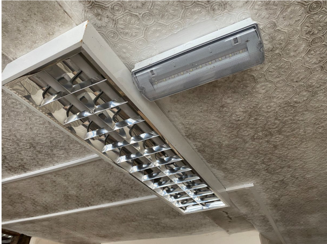
Figure 21: Relatively typical intrusive approach to surface mounted lights of multiple styles, plastic ducted wiring.
