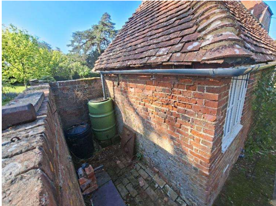
Figure 12 West elevation of the outbuilding showing the eroded brickwork to the upper part of the elevation.
