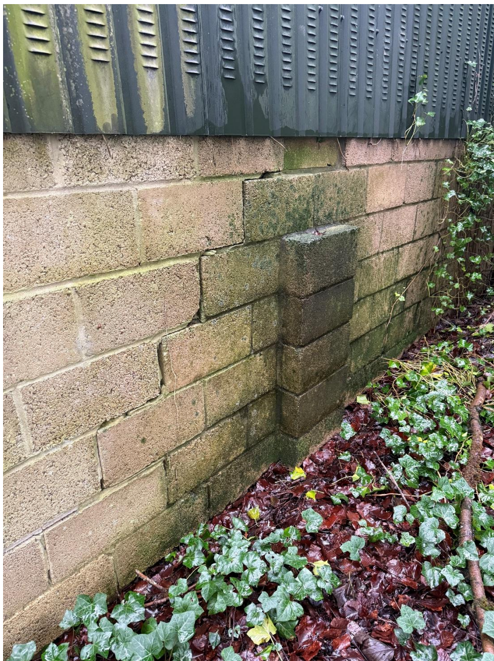
Figure 13: Masonry panel damage
