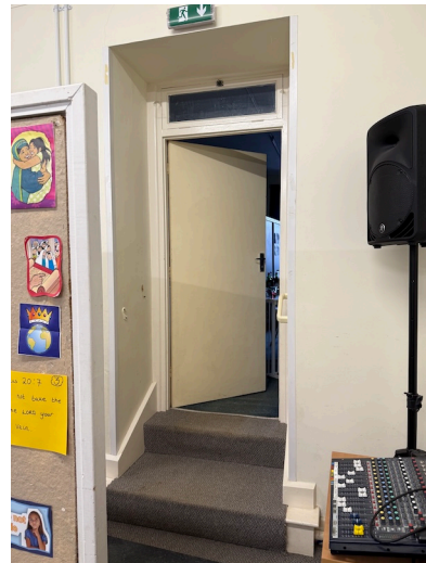
Fig 16 – Narrow Doorway (800mm) with 3 Steps – Accessibility Barrier
