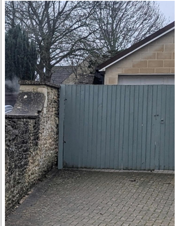
Figure 18: photograph taken to provide matching angle as Google Street View December 2025 This shows the wall is appearing closer to the garage than previously. Confirming recent, ongoing movement.
