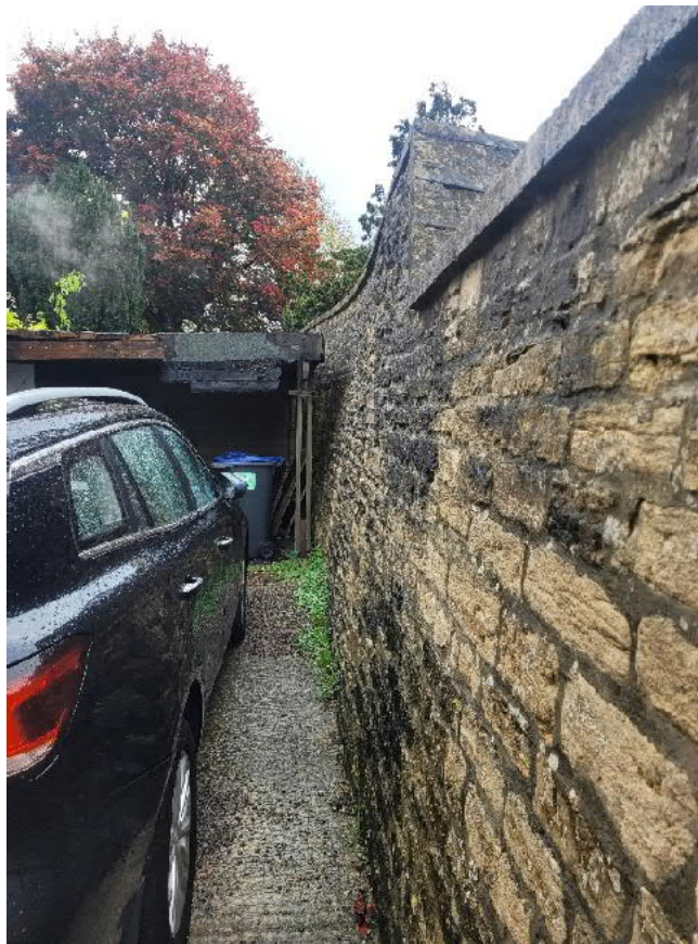
Figure 8; The wall can be seen to follow an S shaped geometry at the base of the wall, however at the head of the wall this geometry is exacerbated as the wall becomes out of plumb.
