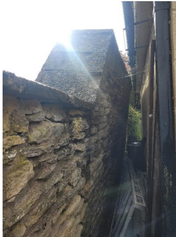
Figure 5; View from front of garage . wall visibly deviates out of Plumb and becomes significantly closer to the garage at its central point.
