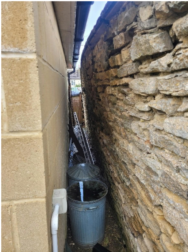
Figure 4: View From rear Garden side, the head of the wall has moved and can be seen to be leaning significantly towards the neighbouring garage. When measured, at lower level the wall is circa 600 millimetres from the garage wall and at eaves level it is circa 300 millimetres from the garage wall. This shows that the wall head has moved approximately 300mm over the years.
