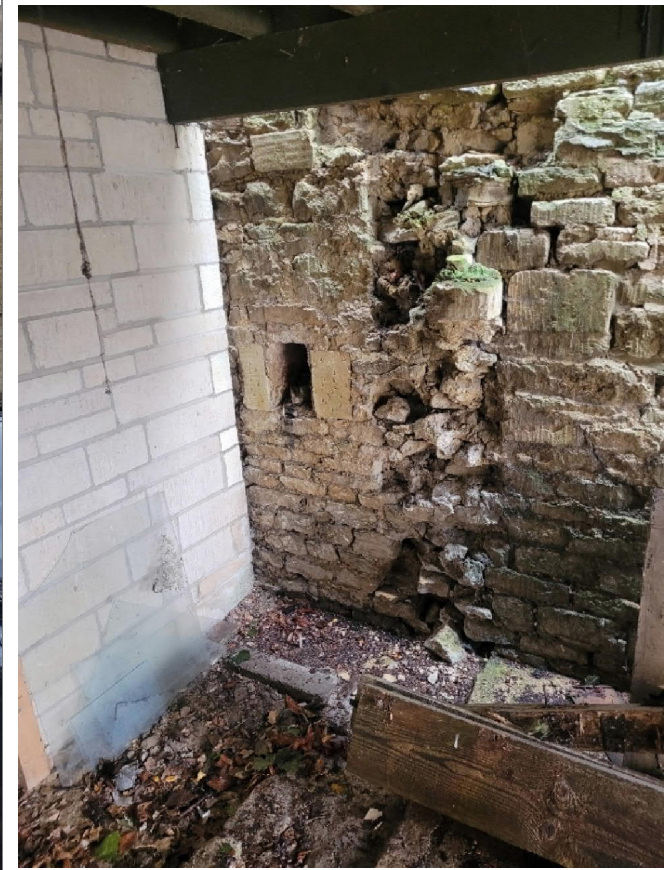
Figure 12; Visible scarring in the wall within the carport shows where a previous buttressing wall has been removed. This has left the rubble exposed and unconsolidated. The out of plumb movement of the wall occurs forwards of this point
