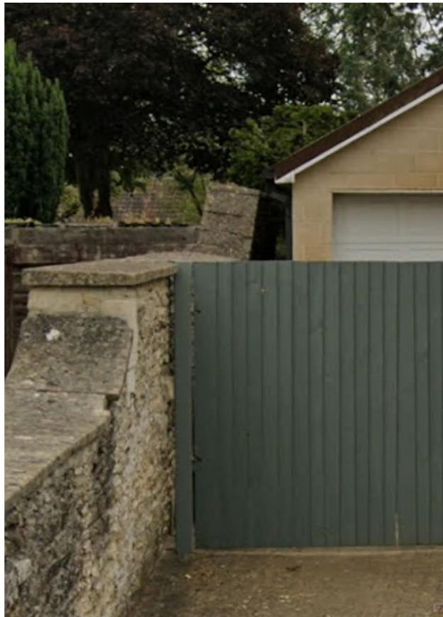
Figure 17; 2024 recent google Street View image showing increased wall incline.
