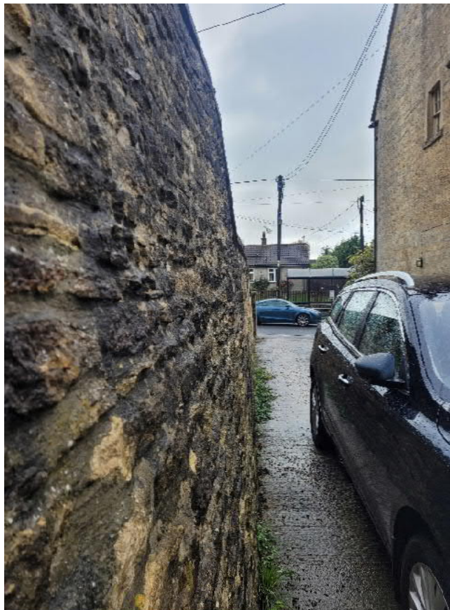
Figure 11; The front section of the wall appears to have been built straight in plan, but has moved to be out of plumb vertically.
