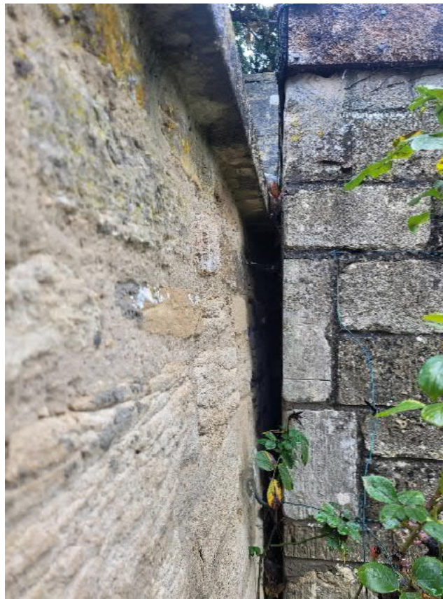
Figure 14; the Garden store does not provide any support to the garden wall
