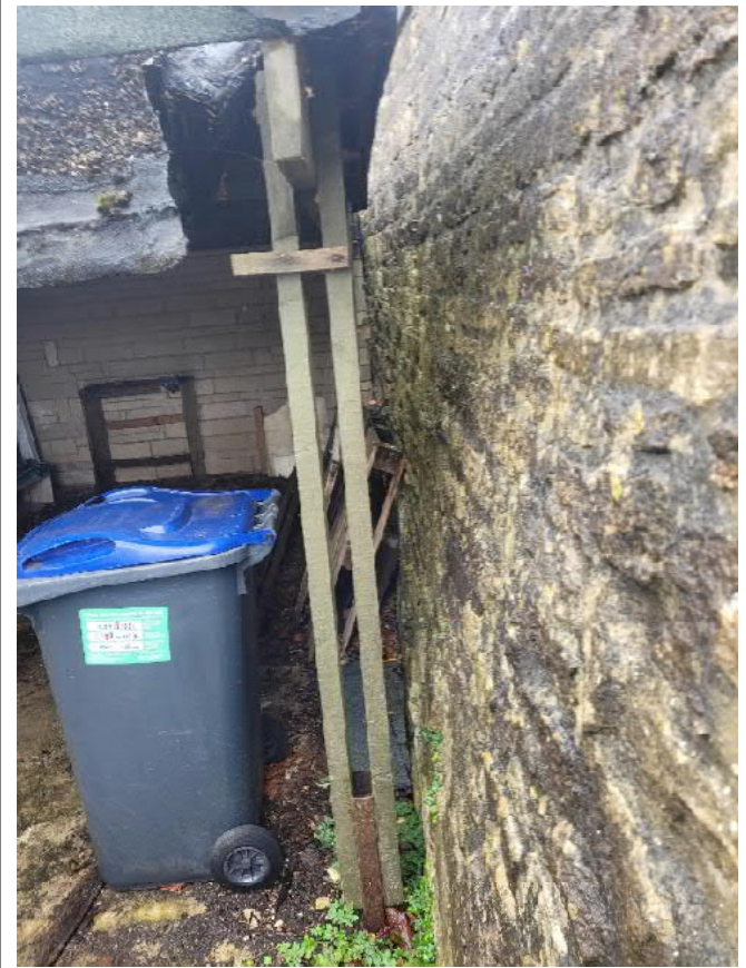
Figure 9; The out of plum geometry of the wall is more significant above 1 metre.
