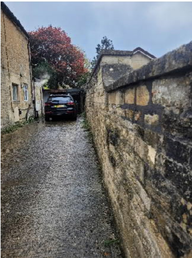
Figure 7: Alongside the driveway at 64 Pickwick Road the wall is low level height of 1.5 metres before it rises to a maximum of 2.75 metres. The out of plum nature only starts approximately in line with the garage, and only rises from the higher ground level.
