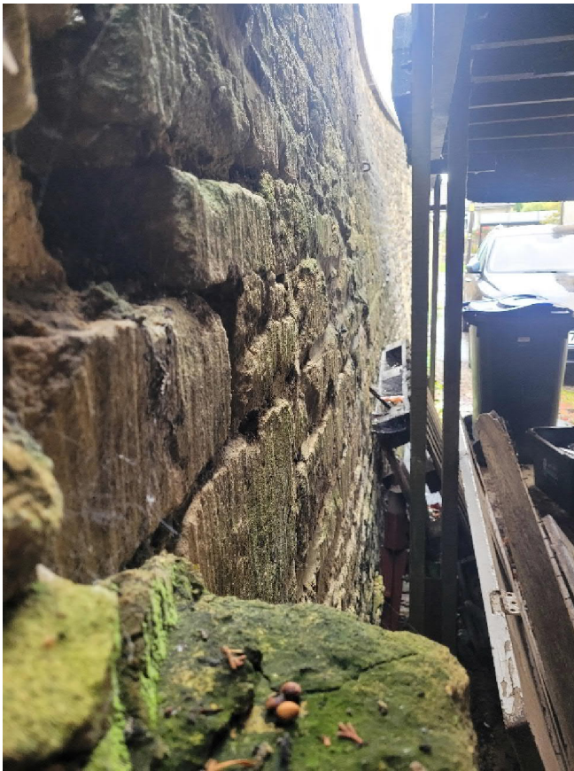
Figure 10; The wall in an S shape on plan and the curvature can be clearly seen. The head of the wall is inclined out of plumb towards the higher ground.
