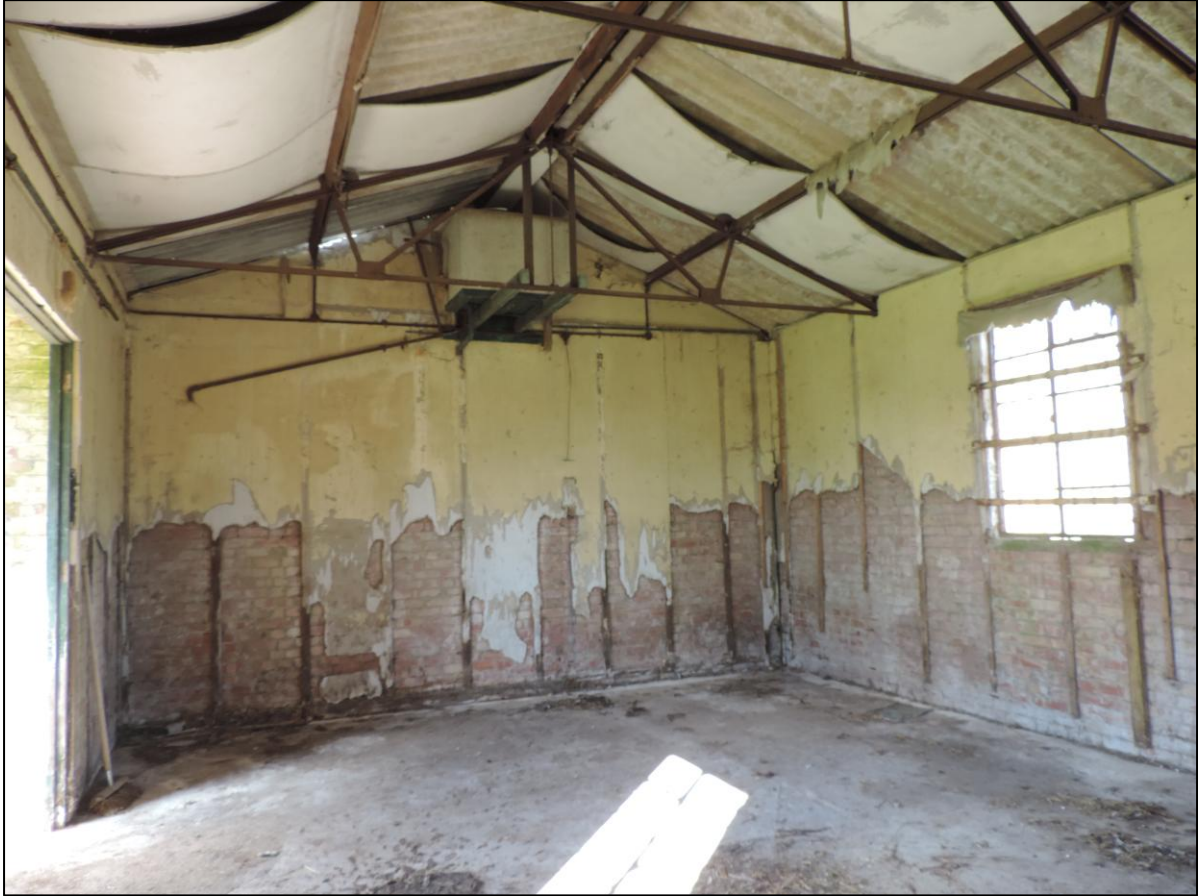
Photo 4 Internal northwest facing view with water header tank in situ.
