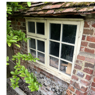
WINDOWS TO BE REPLACED
