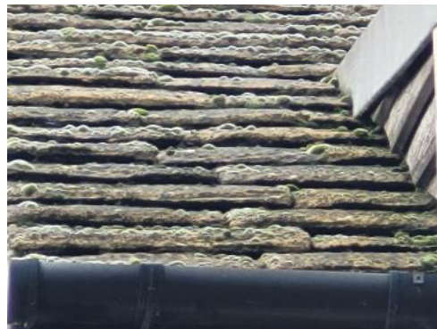
Photo 6: B1 - gaps present beneath the imitation stone tiles.
