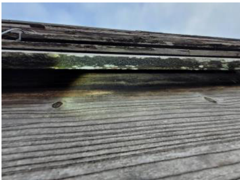
Photo 5: B1 - an example of the gaps present beneath the waney edge timber boards.
