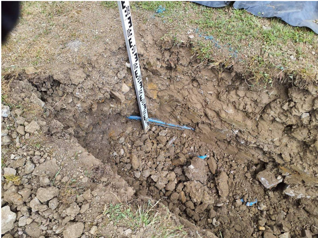
Pipe within larger duct in NW corner.
