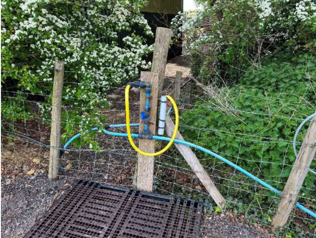
Photo 13: Second water supply point in east corner of Field 1.
