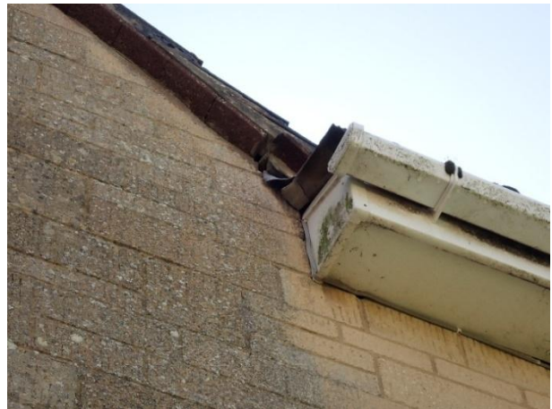
Photograph 6: Gap under flashing on the west elevation end.
