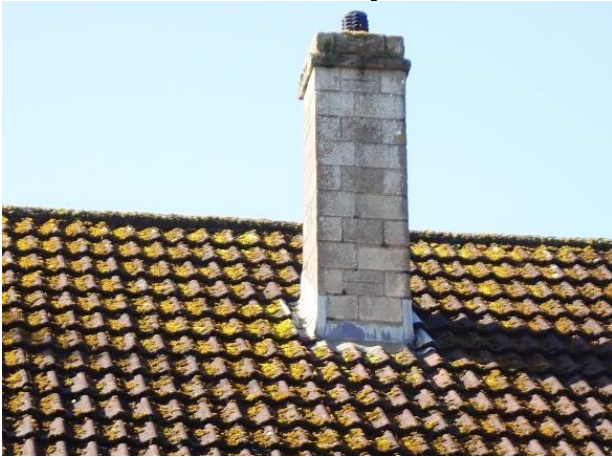
Photograph 3: Lifted lead flashing on C1.
