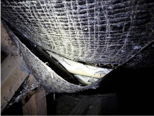
Photograph 13: Internal void, gaps in bitumen felt.
