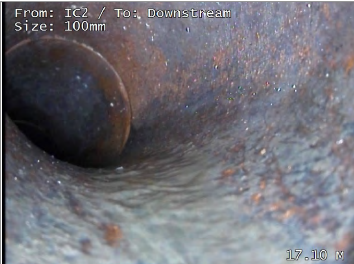
Line of drain/sewer deviates down
