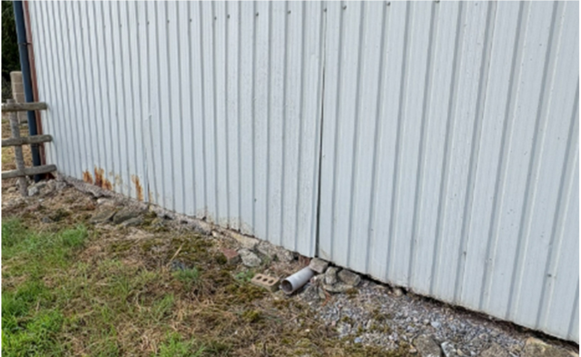
Figure 7. North elevation showing drainage pipe from central slab channel and local washing out of soil beneath slab edge.
