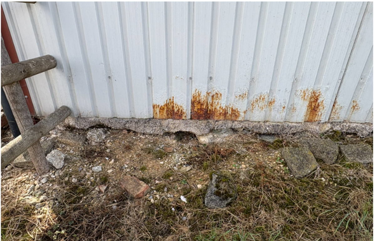
Figure 8. Close-up detail of the same. Slab will require underpinning as part of the conversion works.
