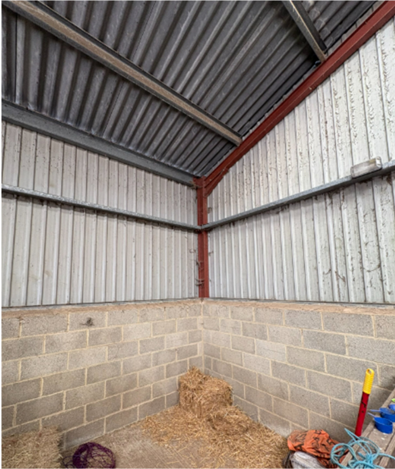
Figure 3. Northwest corner showing cladding rails and blockwork built tight into steel posts.
