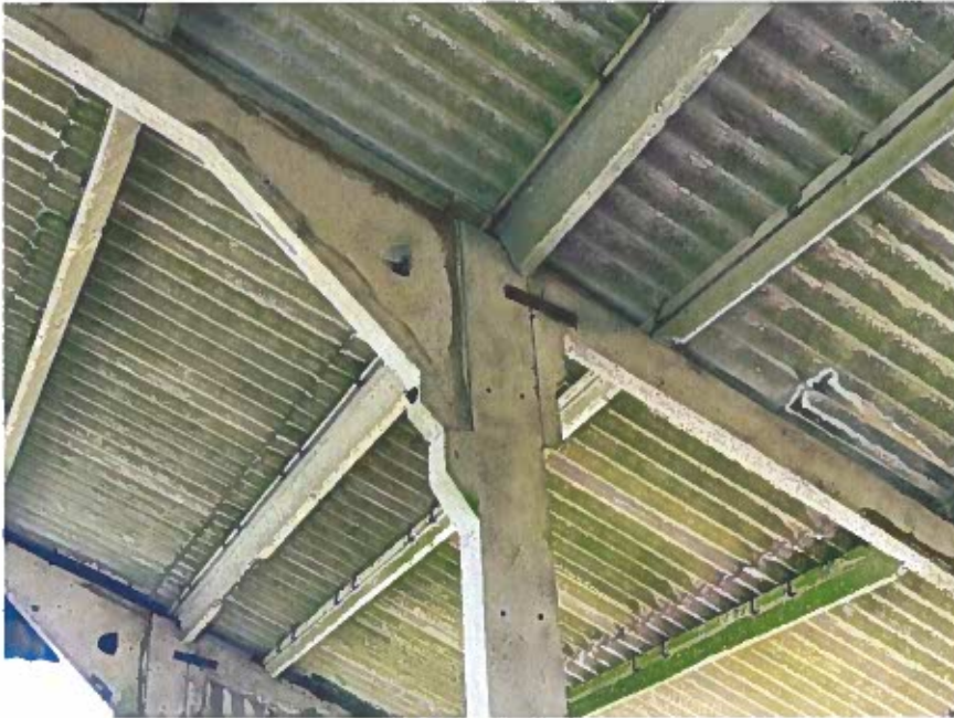
Central Column Head
