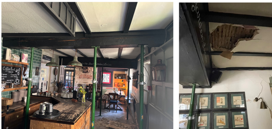
Internal Damage to Beams and Lath and Plaster Ceilings
