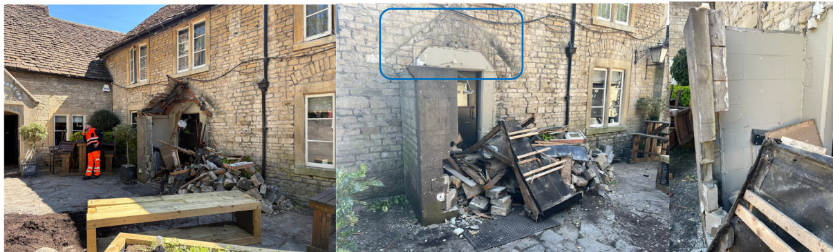
Damage to Porch (Pre-existing Arch Circled in Blue)
