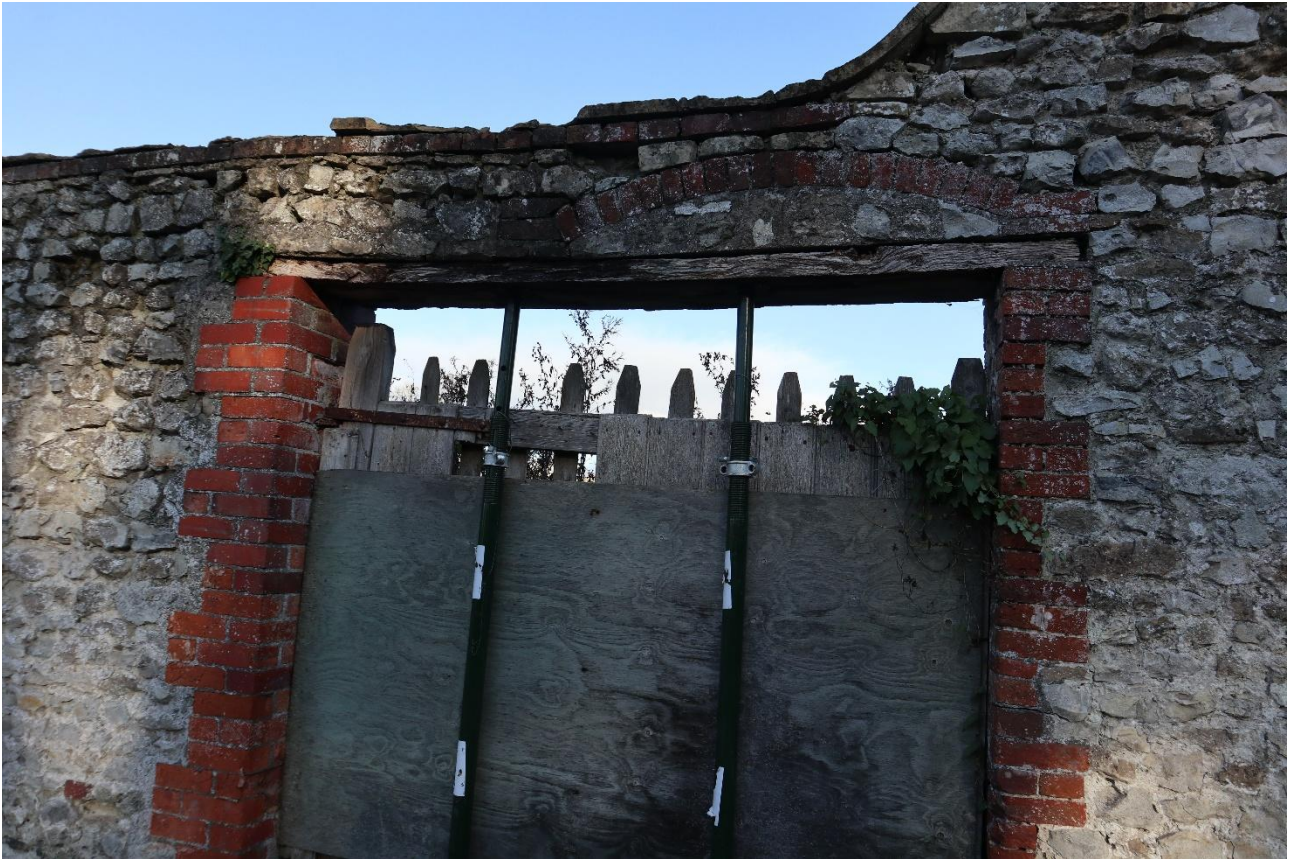
Figure 4 Image showing the poor condition of the blocked entrance within the Boreham Road Boundary wall to the west of The Cotes (Grade II).
