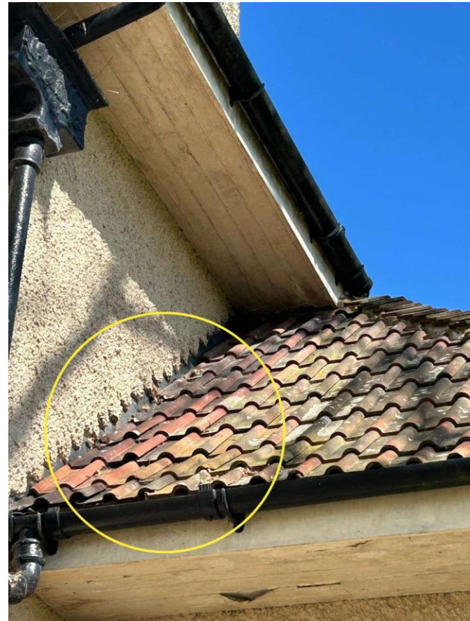
Lifted roof tiles present on the small extension to the east.
