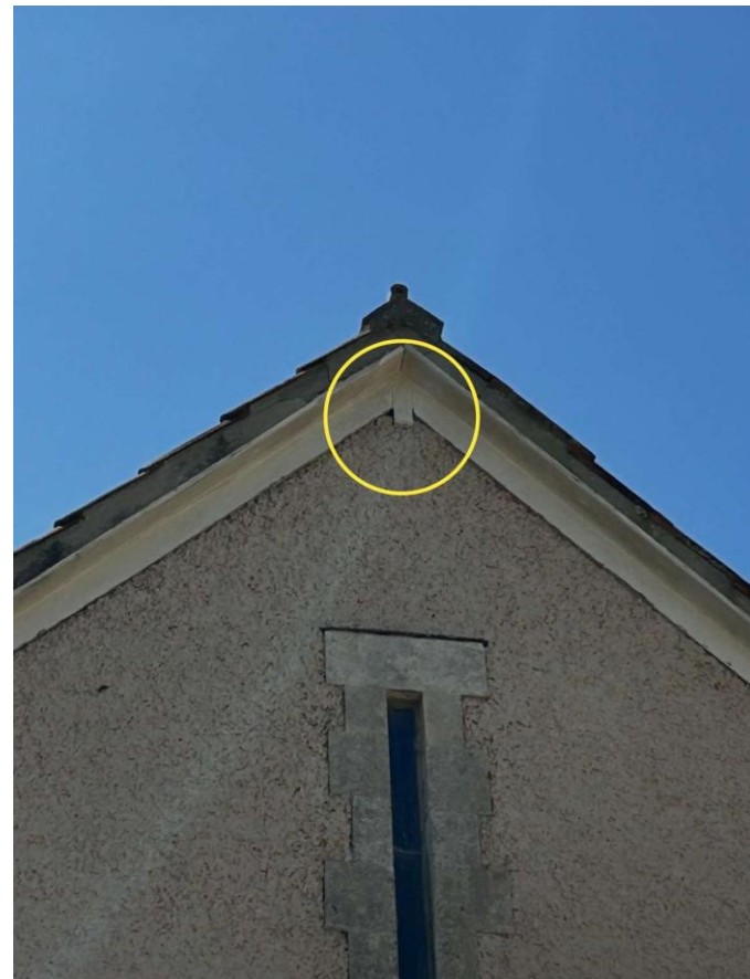
Gap behind the bareboard on the northern gable end.
