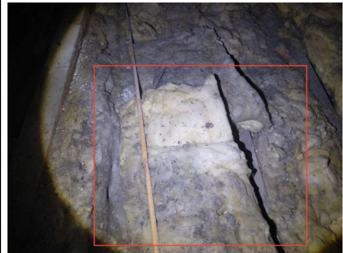
B1 - Loft void LV1 bat droppings
