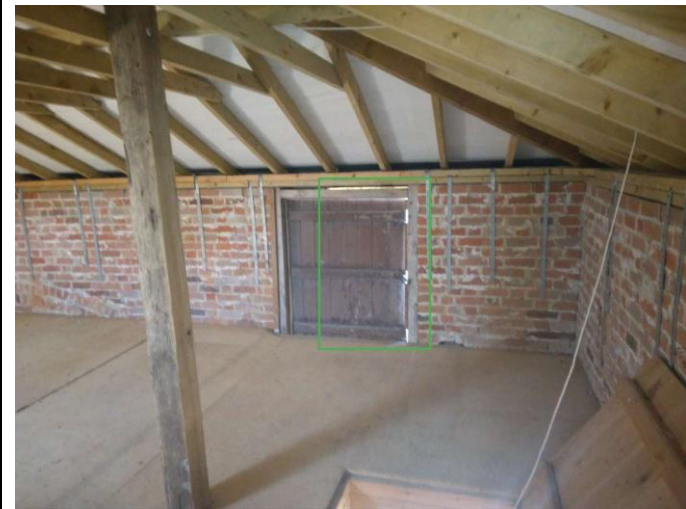
B2 - Gaps between the door and frame
