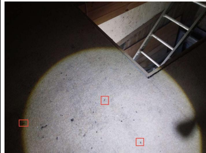
B2 - Bat droppings in B2
