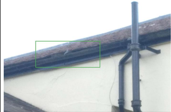
B1 - Lifted tiles on the western elevation
