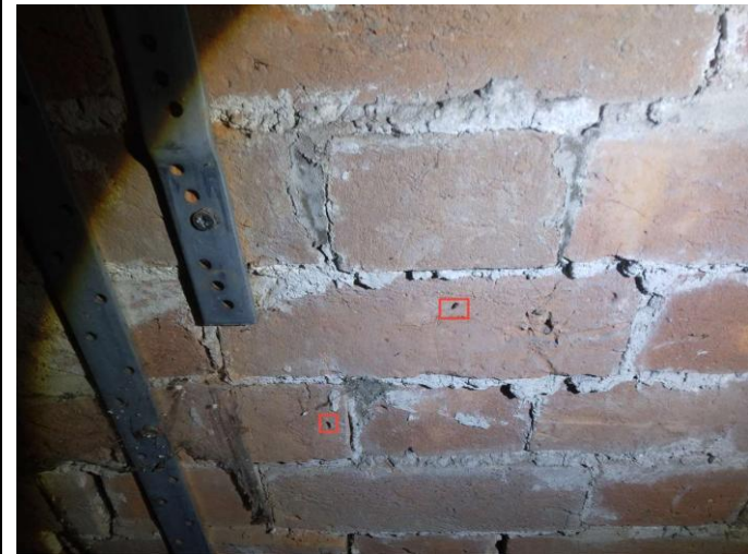
B2 - Bat droppings in B2
