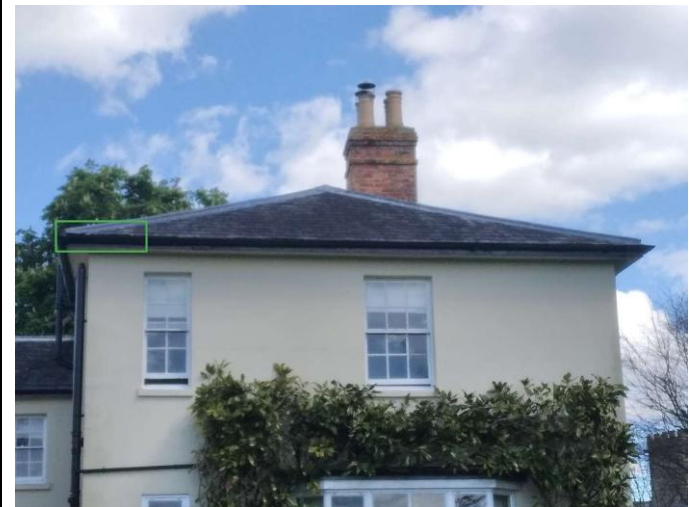
B1 - Lifted tiles on the southern elevation
