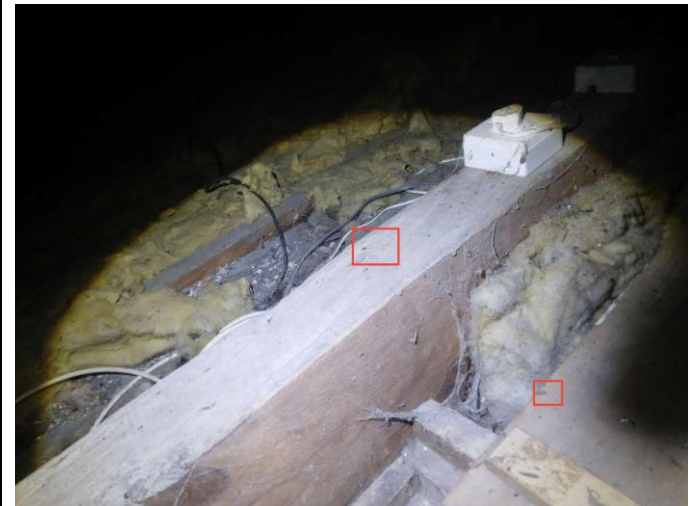
B1 – Loft void LV1 bat droppings
