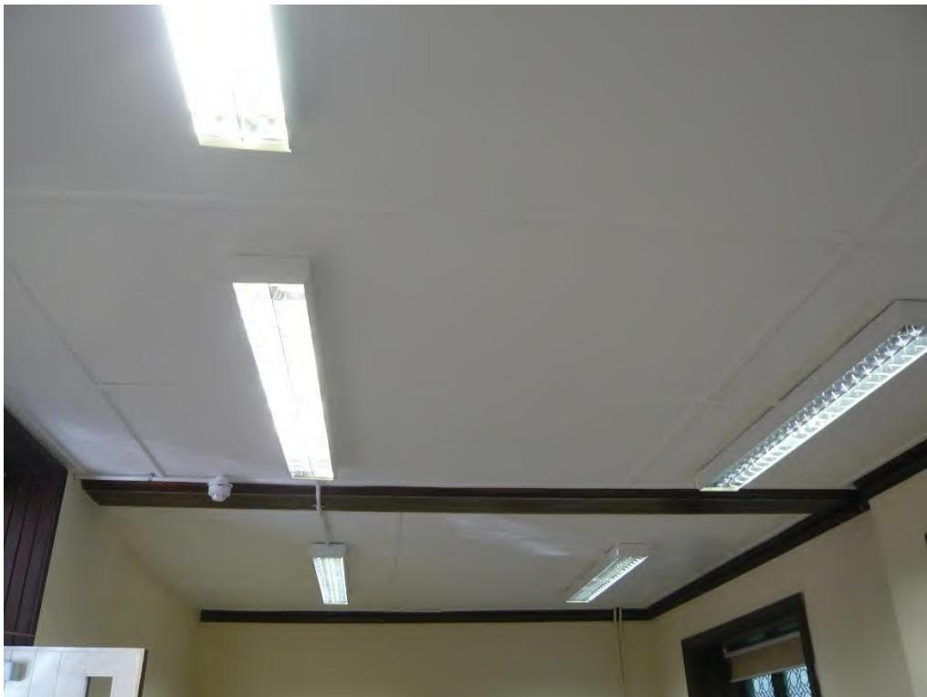
Fig.25 Suspended ceiling and strip lighting in W Range
