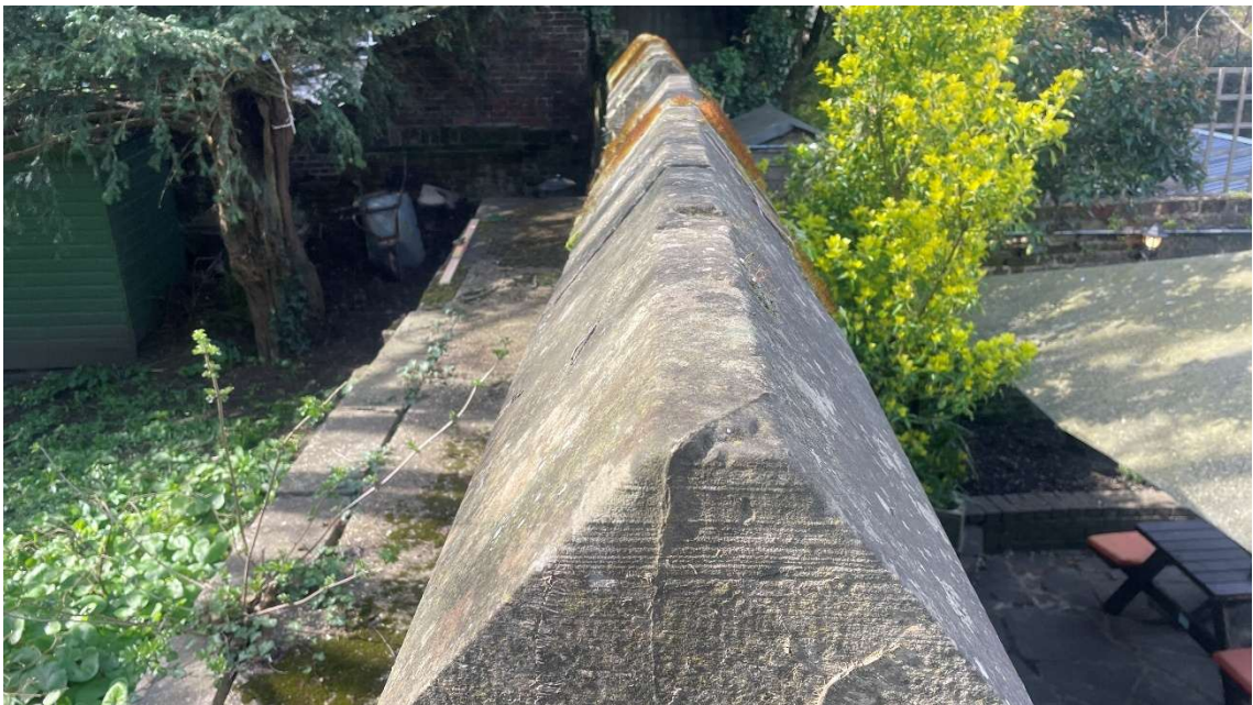
Figure 3.9i: Deviation in the wall head indicating the northwards movement of the wall
