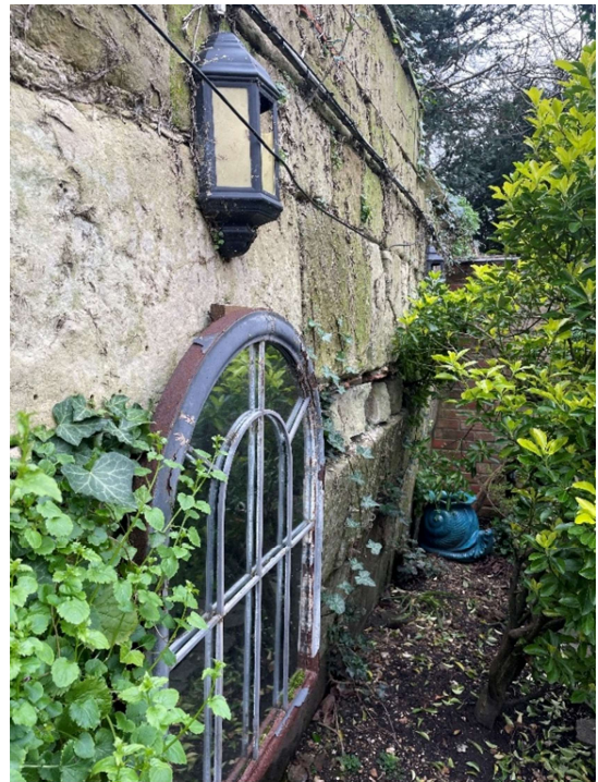
Figure 3.13c: Loose stonework is evident at low level
