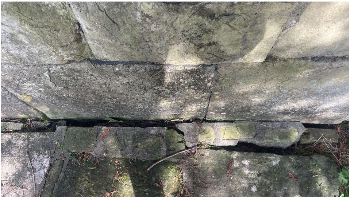
Figure 3.4b: Gaps between the wall walk and crenellated parapet section allowing water and root penetration
