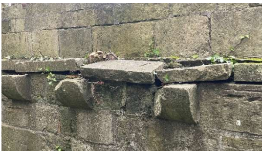
Figure 3.9a: The wall walk paving collapsing locally
