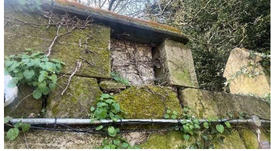
Figure 3.14d: Missing stonework at crenellation level
