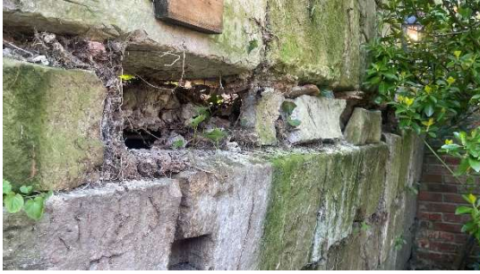
Figure 3.14c: Missing stonework in the wall
