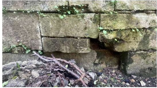
Figure 3.14f: Missing stonework at low level
