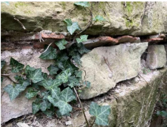
Figure 3.14a: Loose stonework in the wall
