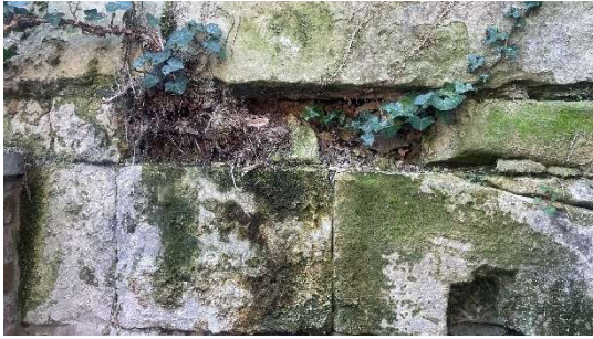
Figure 3.14e: Ivy growing from the wall
