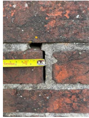
Figure 27 – Close view of typical south elevation separation crack
