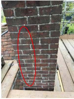
Figure 26 – Separation cracks at south elevation
