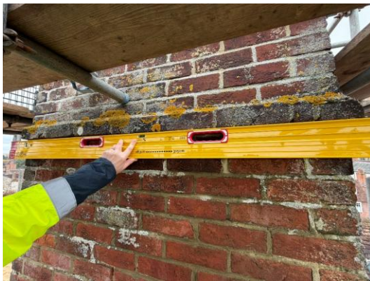
Figure 37 – 10mm string course dip at west
