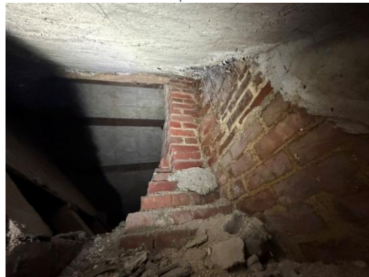
Figure 29 – Base of stack within roof space
