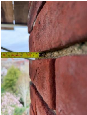
Figure 13 – Typical depth of pointing loss
