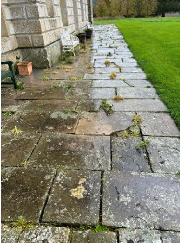
Fig.15 Damaged area of paving by the south side of the house
