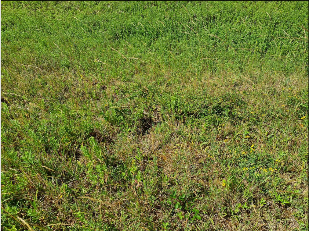
Site Walkover 26.06.2025: Cracks due to possible desiccation located on the slope (Facing North)
