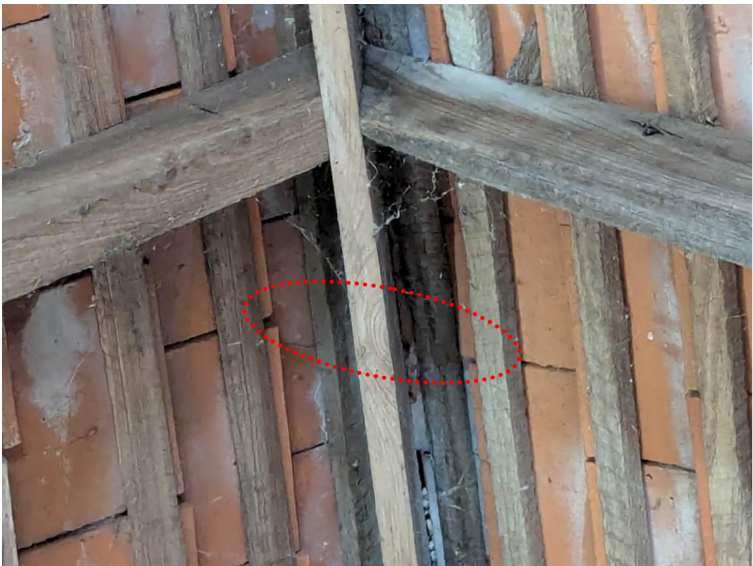
Photo 9/10 The Old Livery, (south aspect) tile clay roof tiles and high potential feature tile gaps below ridge.
