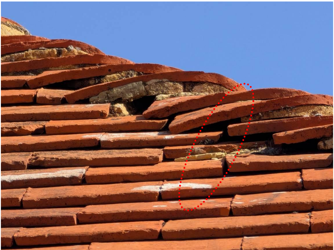
Photo 5/6 The Old Livery, (south aspect) tile clay roof tiles with access gaps.
