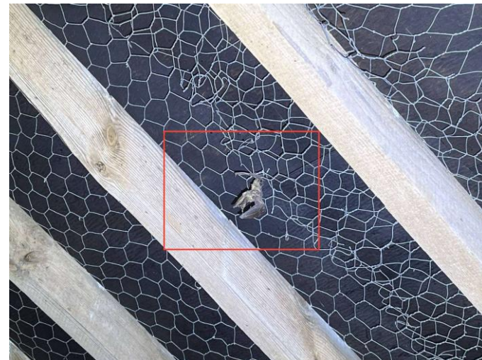
Dead brown long-eared bat inside the loft void of B2.
