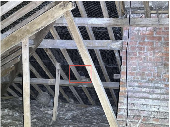
Tear in roof lining B2.
