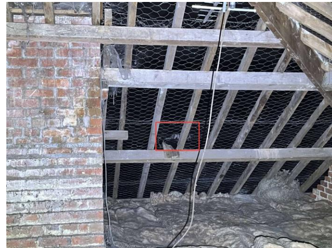
Tear in roof lining B2.
