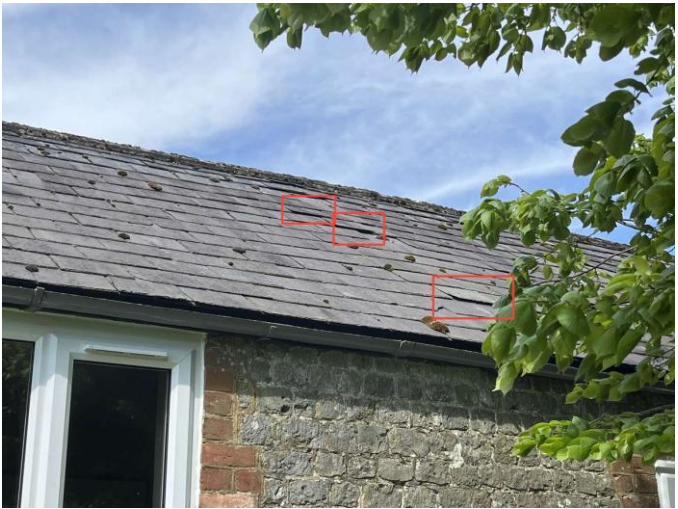
Lifted roof tiles on the east elevation of B1.
