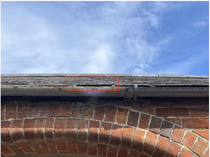
Lifted roof tile on the edge of the west elevation of B1.
