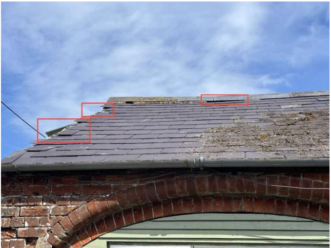
Slipped, lifted and missing tiles on the southern elevation of B1.
