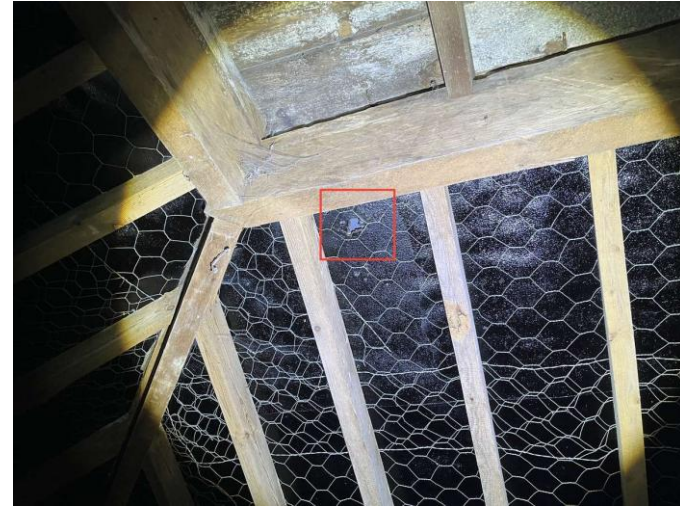
Tear in roof lining B2.
