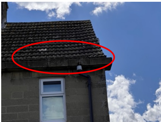
Photograph 18: Lifted roof tiles.
