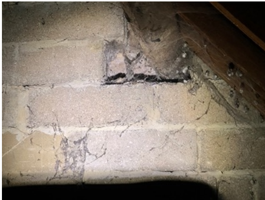
Photograph 16: Gap in the wall.
