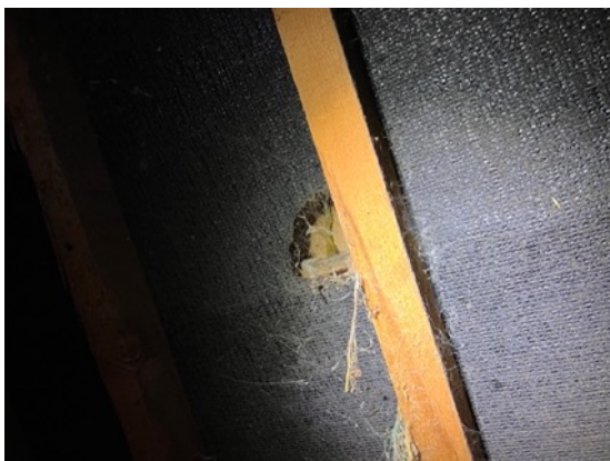
Photograph 14: Hole in the roof lining.
