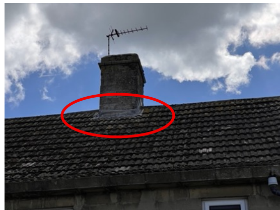
Photograph 19: Raised lead flashing.
