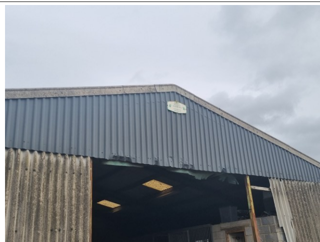
Photograph 7. Permanently open access to the building.
