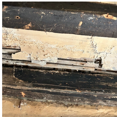
GF – Beams showing sign of decay
