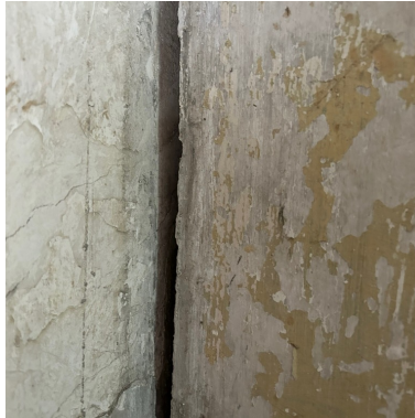
FF008 – Wall detached from exterior
