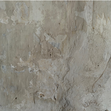
FF001 – Wall lime plaster
