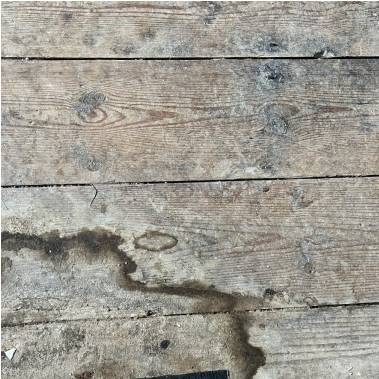
FF02 – floor / pine showing sign of decay
