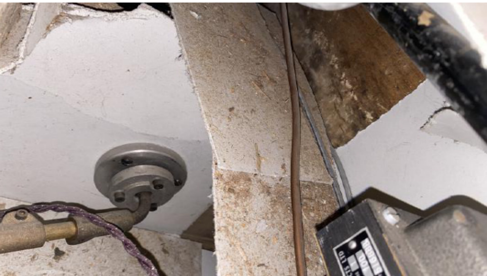
Damaged textile paper to boxing, joist cladding & top of dropped ceiling to Salon
