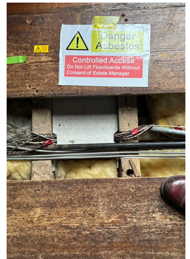
Lining panels containing asbestos (Ground Floor)
