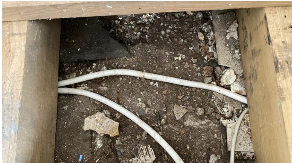
Asbestos containing tile used as packers below floor joists
