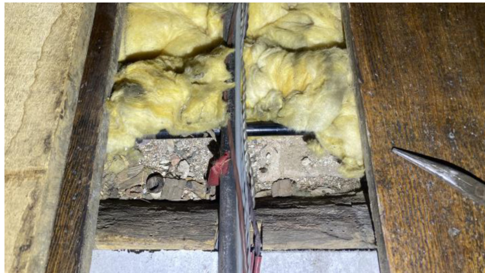
Board dust/debris containing asbestos
