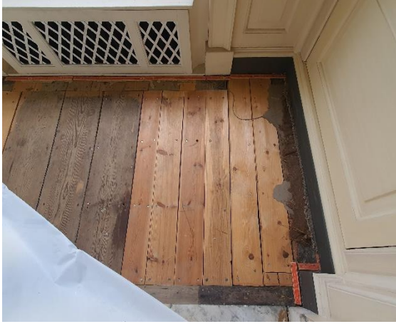
Figure 24: : Exposed timber floor slats after the removal of the carpet – Chinese Bathroom FR04
