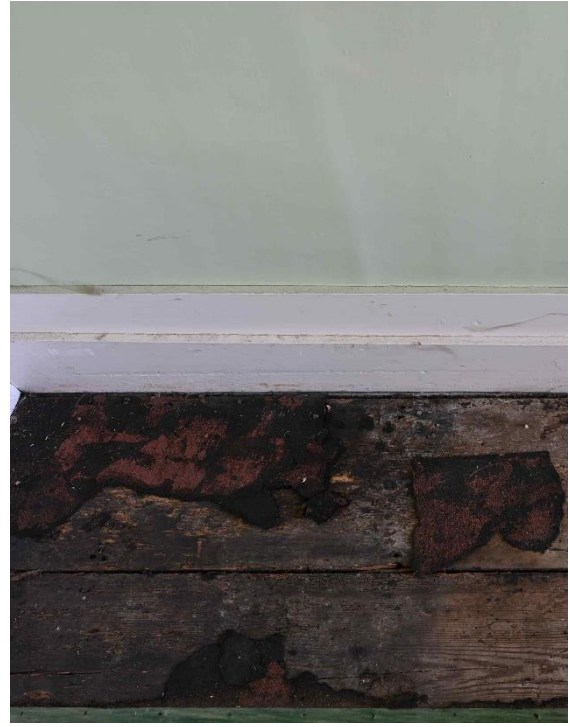
Figure 94: Adhesive from the vinyl on existing timber boards - Staff Bathroom SR17
