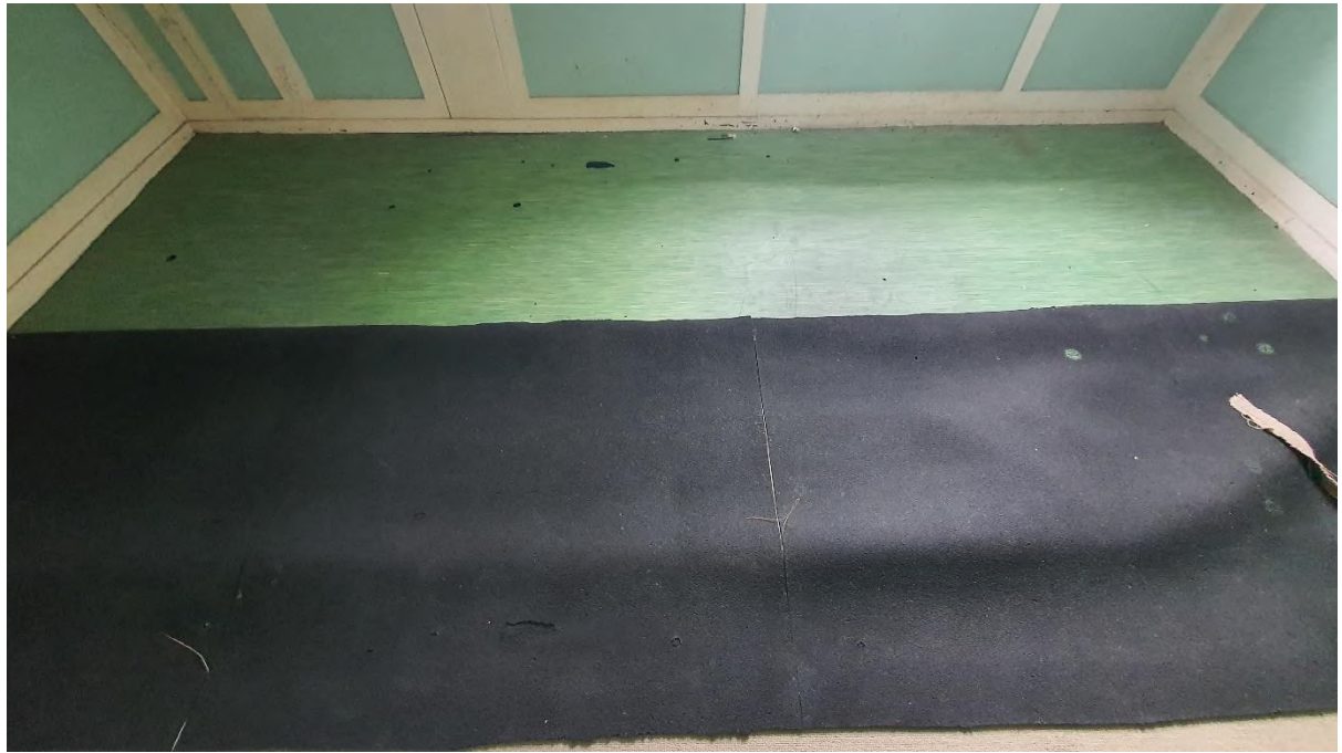
Figure 79: Floor - removal of carpet and exposing the vinyl - Staff Bathroom SR14
