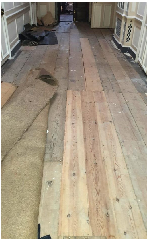
Figure 62: Timber boards post carpet removal - Corridor FR11
