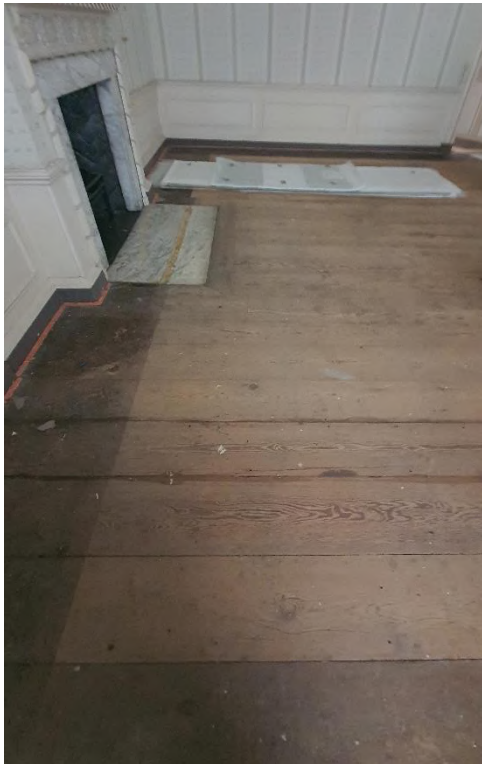
Figure 77: Timber boards, post carpet removal - Mrs. Hyams Bedroom FR12
