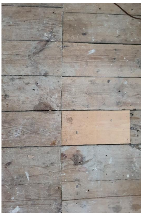
Figure 89: Old timber repair to floor - Mr. Hyams Bathroom FR14
