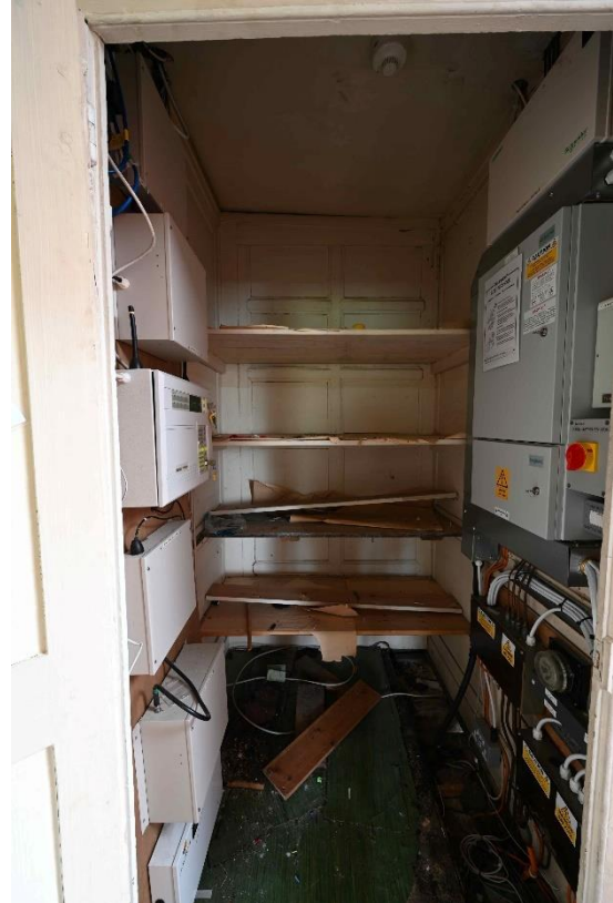
Figure 106: Alarm Cupboard SR21
