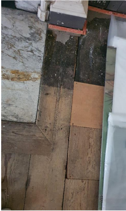
Figure 75: Old floor repairs - Mrs. Hyams Bedroom FR12
