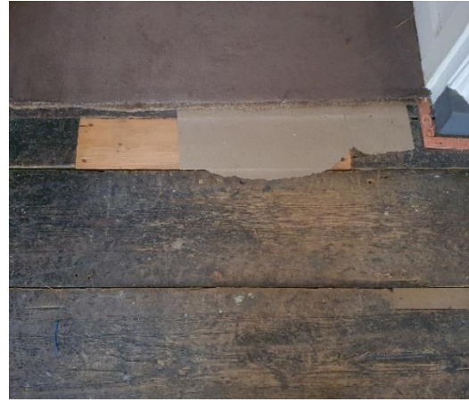
Figure 30: Old repair to floor - Pink Bedroom FR05
