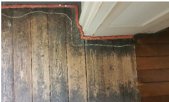
Figure 7: Floorboards by door threshold - Library
