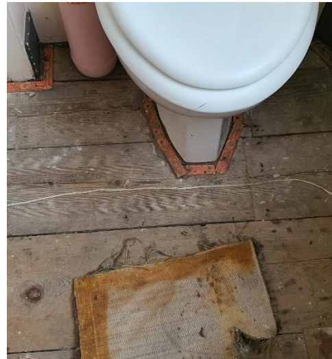
Figure 37: Timber boards, post carpet removal - Pink Bathroom FR06
