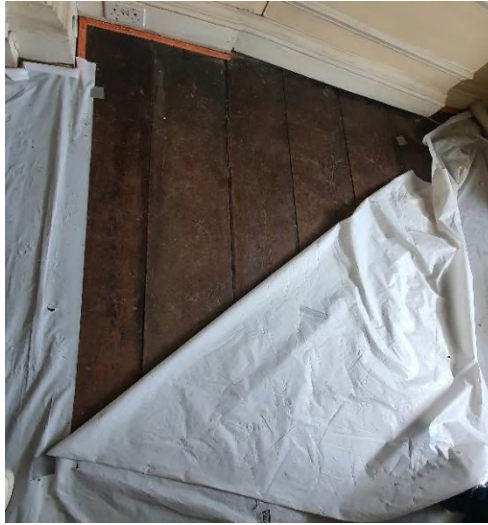
Figure 18: Small inspected part of the timber - Chinese Bedroom FR03
