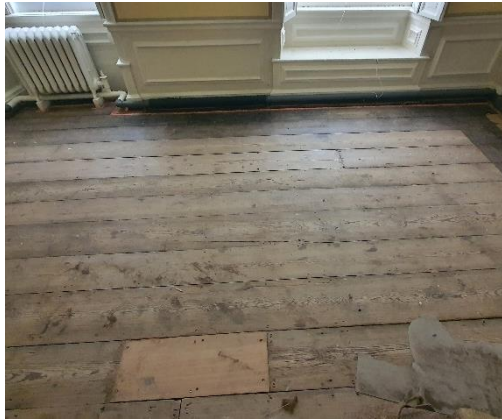
Figure 55: Timber boards post carpet removal – Yellow Bedroom FR09
