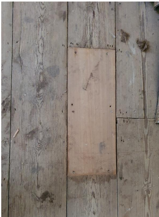
Figure 57: Old timber repair to floor - Yellow Bedroom FR09
