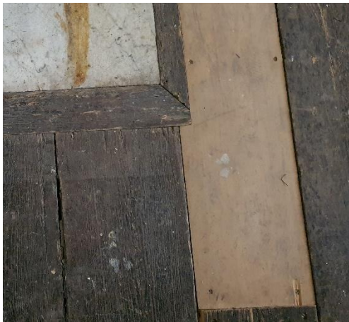
Figure 31: Old repair to floor - Pink Bedroom FR05
