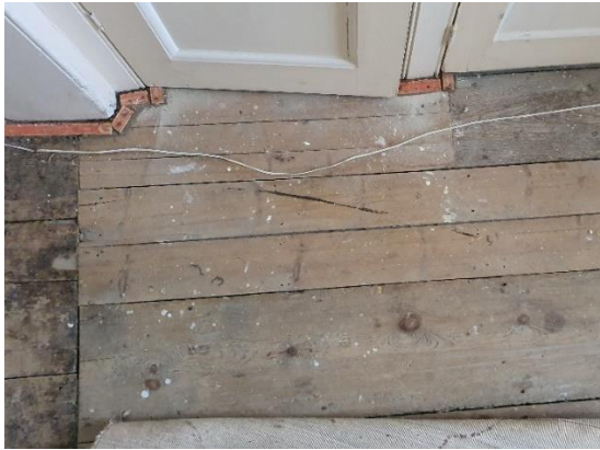
Figure 36: Timber boards, post carpet removal - Pink Bathroom FR06
