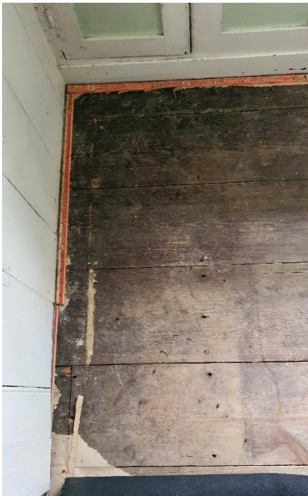
Figure 74: Timber under carpet - Sewing Room SR13
