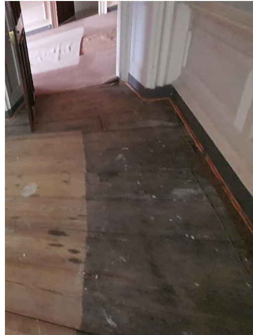
Figure 83: Perimeter timber boards - Mr. Hyams Bedroom FR13
