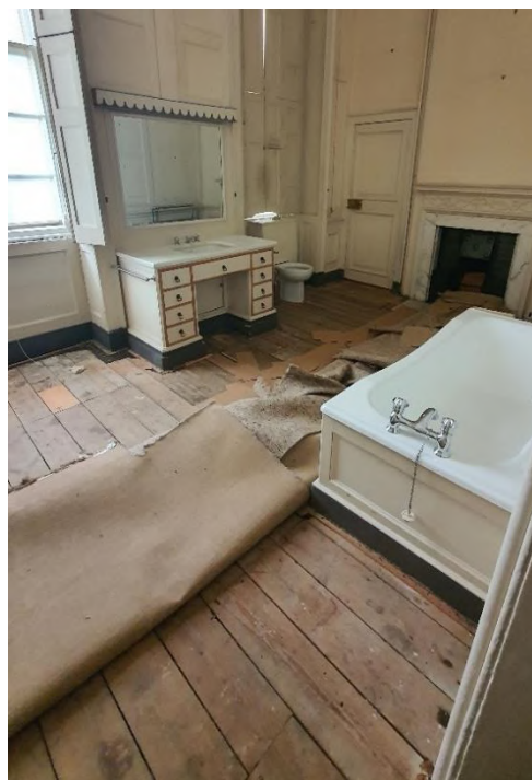
Figure 90: Timber boards, post carpet removal - Mr. Hyams Bathroom FR14
