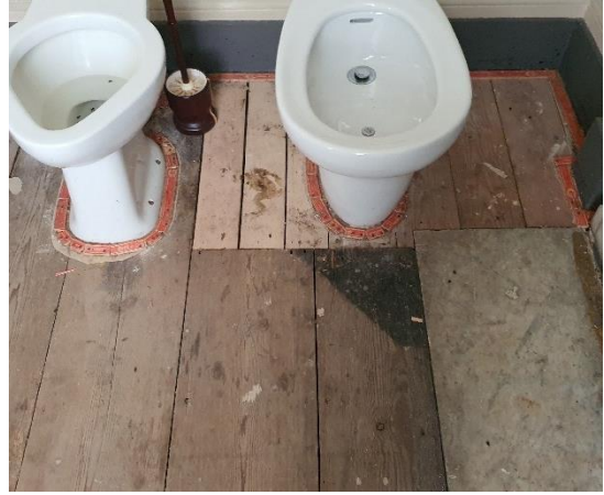
Figure 6: Timber floor old repairs - Blue Bathroom FR01
