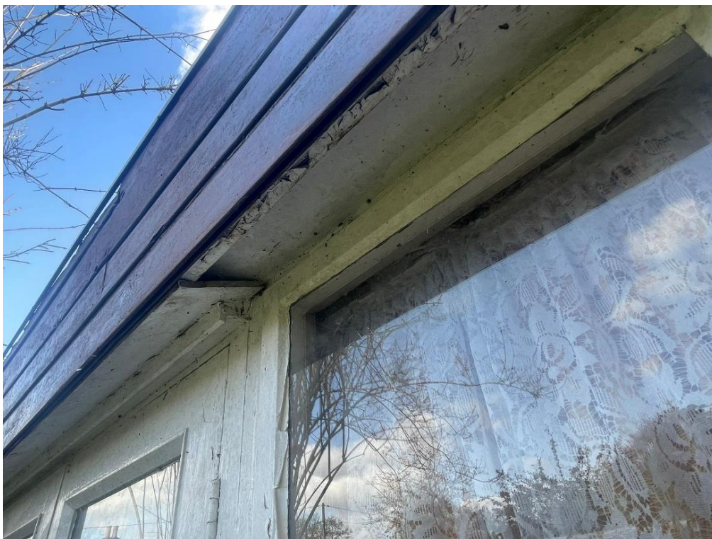
Photograph 4: Gap between soffit sections
