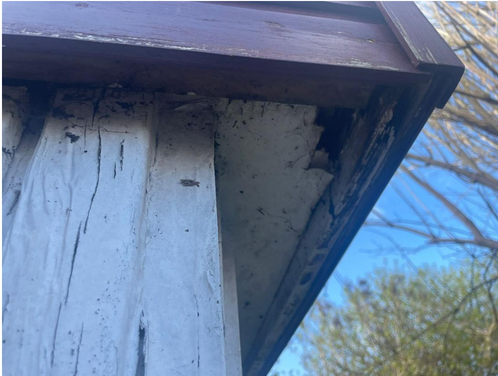
Photograph 3: Timber rot within soffit on eastern elevation
