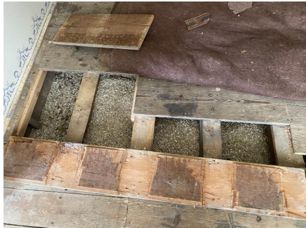
Loose fill vermiculite insulation
