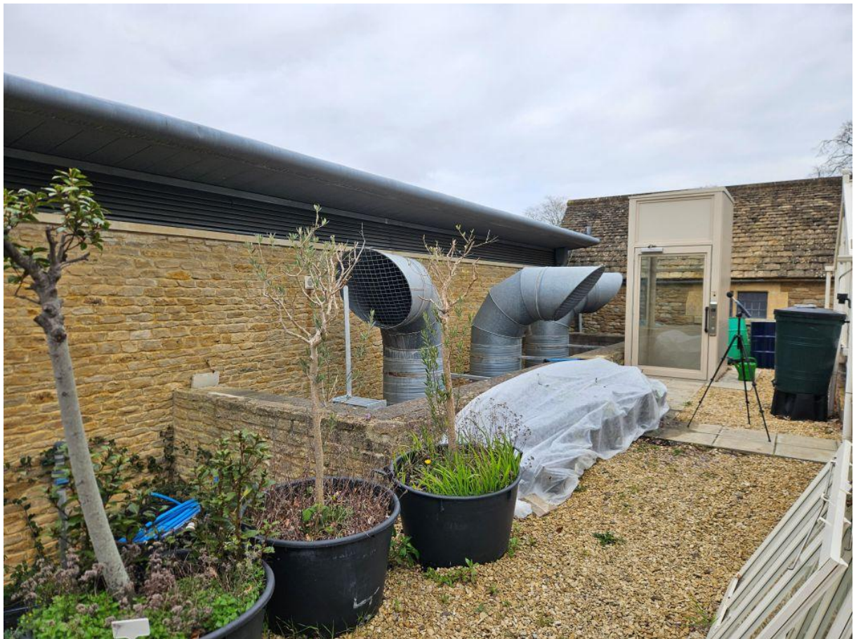
Figure 4: Photo of three exhaust cowls above the AHU ventilation trench (looking north).
