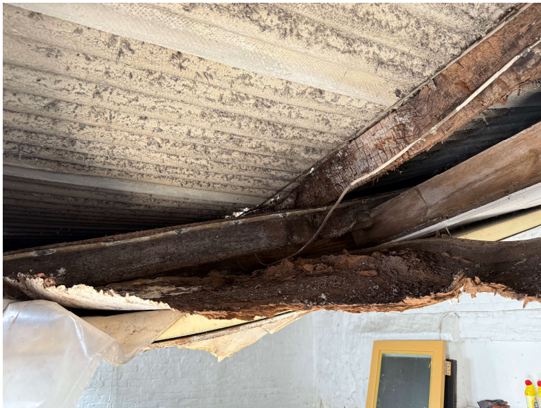
Internal image of store roof to be replaced
