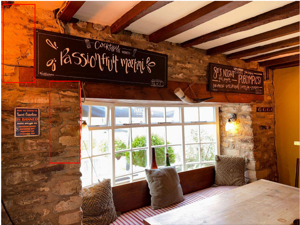
Picture 12 - Vertical to stepped crack below the timber lintel to Area 2 on the main property
