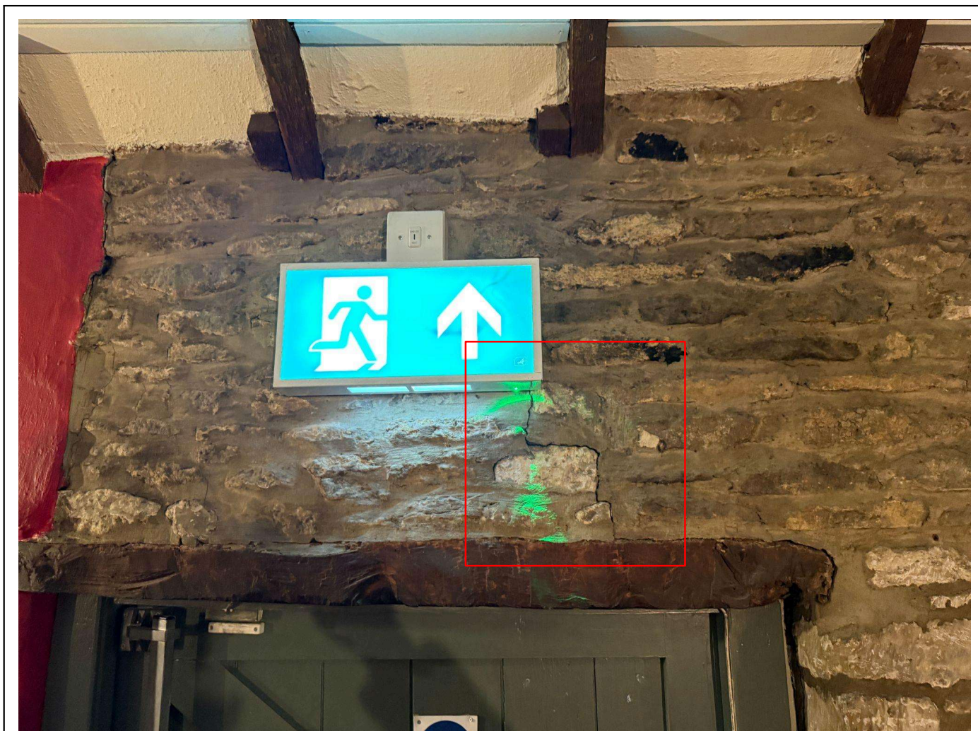
Picture 8 - Stepped crack below the fire exit sign on the south wall of the Dining Area
