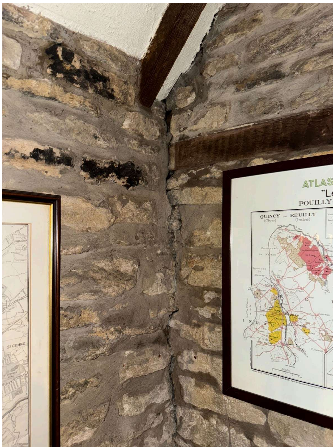
Picture 10 - Vertical cracks to the lefthand corner of the gable wall
