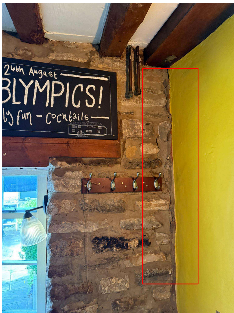
Picture 13 - Vertical crack adjacent to the timber lintel to Area 2 on the main property.
