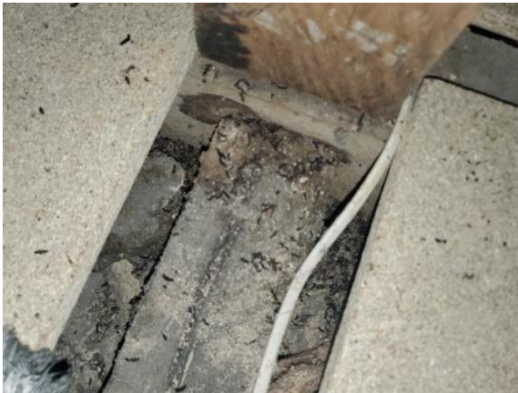
Photo 9: Concentration of bat droppings discovered within southern loft void.
