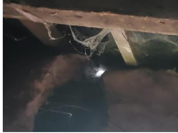
Photo 8: Daylight ingress at the eaves within southern loft void.
