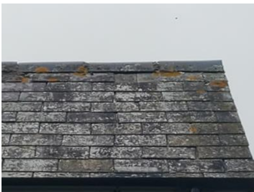
Photo 5: Gap beneath ridge tile at the southern extent of the roof.
