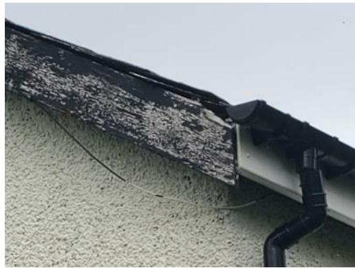
Photo 4: Damaged bargeboard at the south facing gable end.
