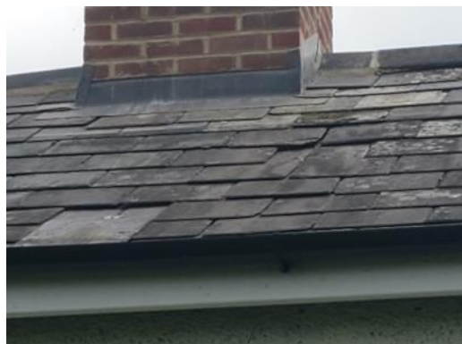
Photo 6: Missing tiles on the west facing roof slope.
