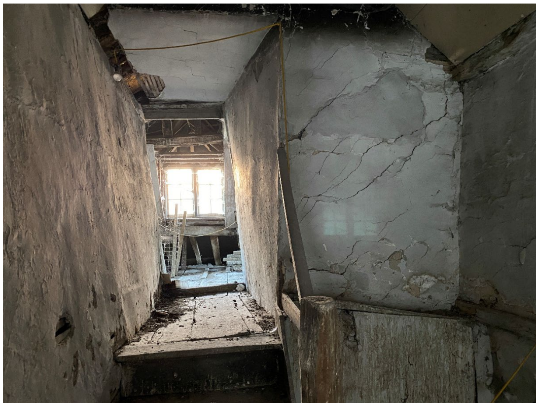
Figure 44: second floor passage from stair to attic, floor will be repaired and levelled, and stair rebuilt, but the misaligned walls will be retained and repaired without straightening to vertical.
