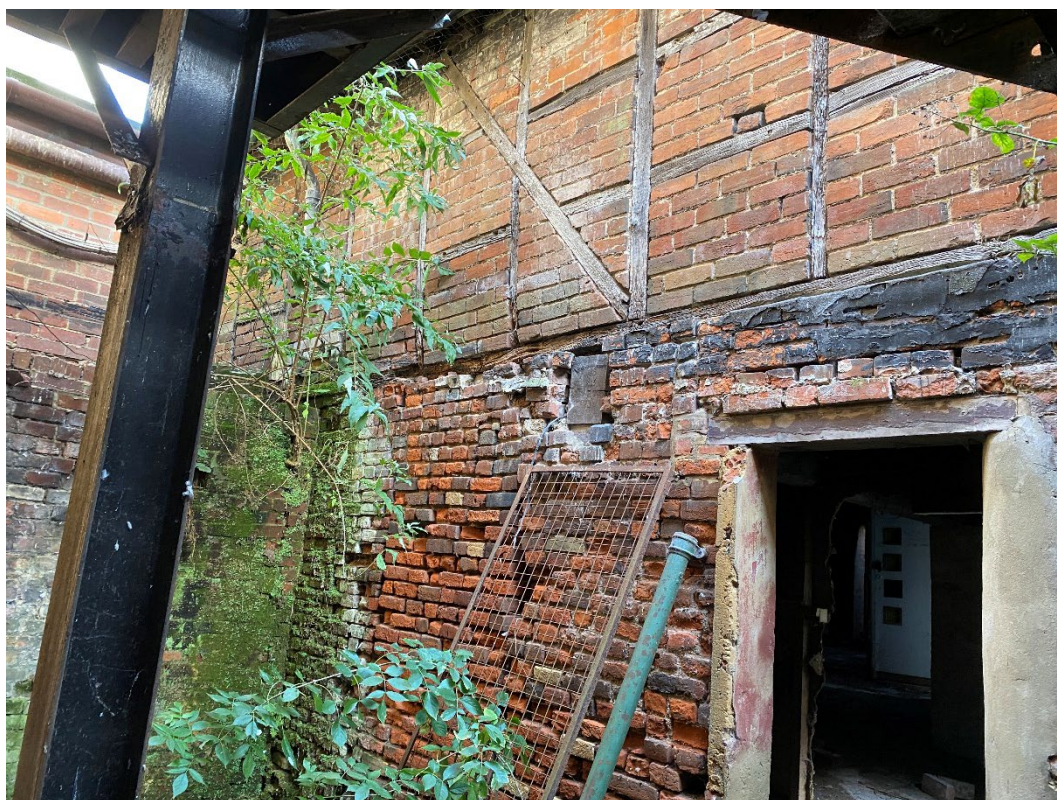
Figure 45: the ground floor possibly 18 th century brickwork much corroded and fragmenting with almost no pointing surviving. Note concrete/cement inserted door on the right, and later brickwork in slender timber frame above – probably 19 th century.
