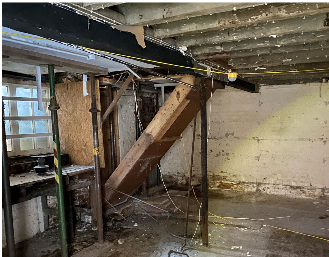
Figure 33: recent ladder stair inserted in the 19 th century stair. Note also extensive propping of northern floor structure linked to adjacent façade decline and collapse.
