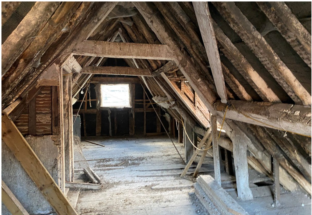
Figure 24: 16 th /17 th century roof structure, frequent later bracing of several periods suggests long structural issues.
