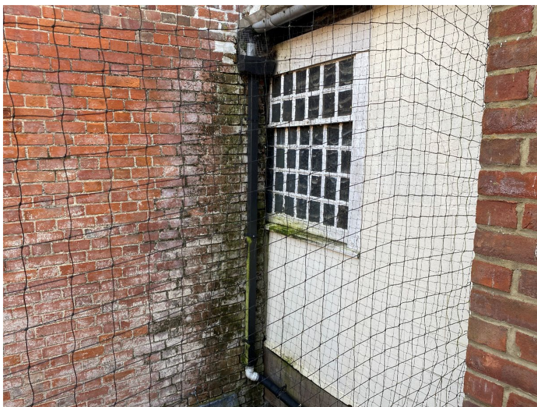
Figure 41: Multi pane 16 over 32 sash to be repaired and relocated so that it is not overlapped by the adjacent brickwork and drainage.
