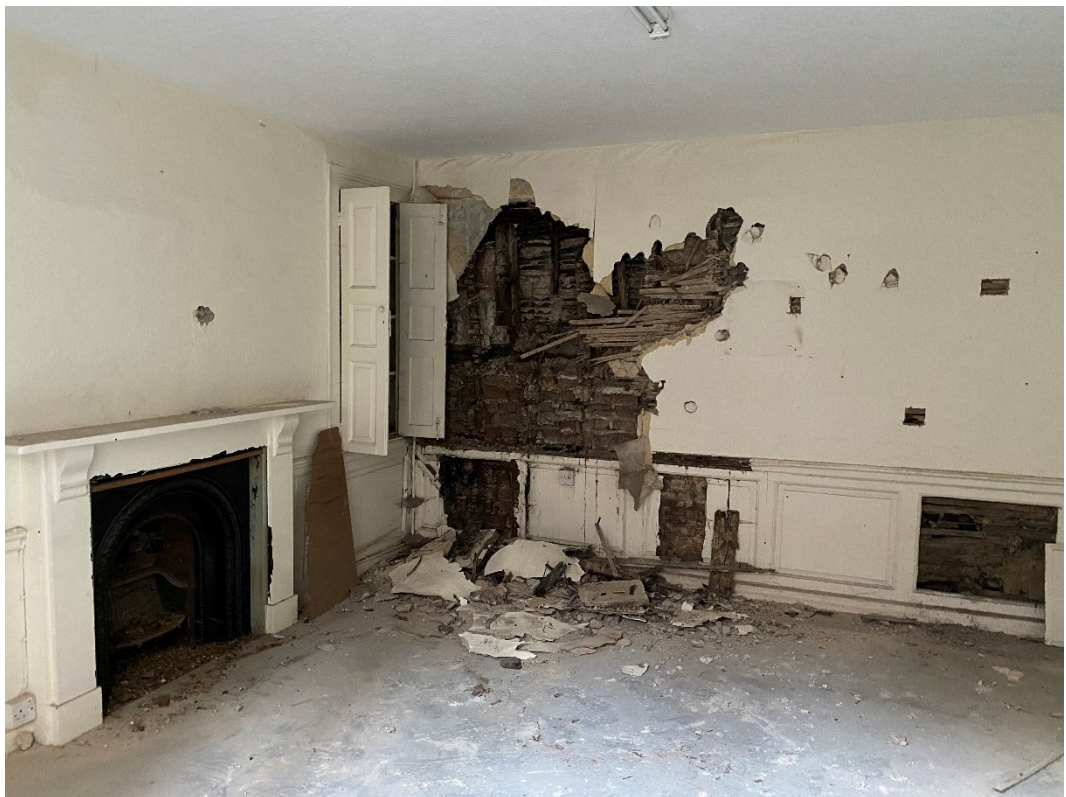
Figure 15: First floor central room off stair half landing with 18 th century dado panelling but older timber frame visible in damaged wall (the result of vandalism).
