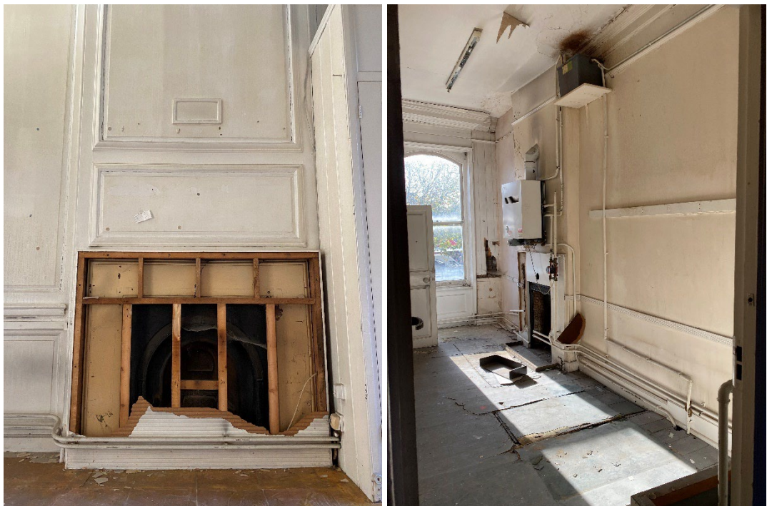
Figure 18-19: first floor spaces, retained fireplaces, panelling, joinery and cornices but run down with unsympathetic later insertions of services.
