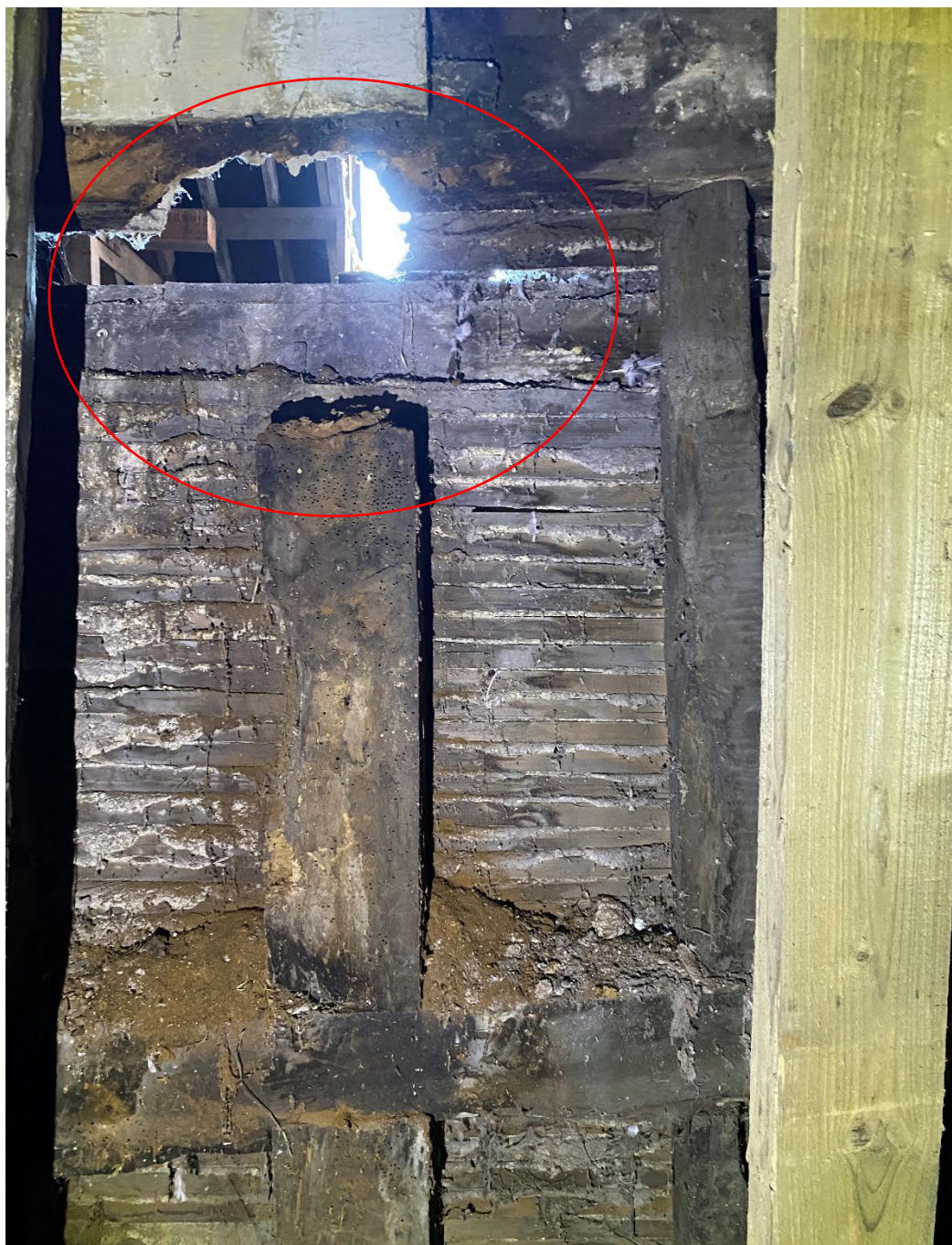
Figure 32: Detail from exposed timber frame showing complete loss of structural detail at joint – the architectural evidence and illustration of this structural element is gone, the timber shown here has since collapsed fully out of the wall. Other similar examples of this level of decay are found throughout the central building.
