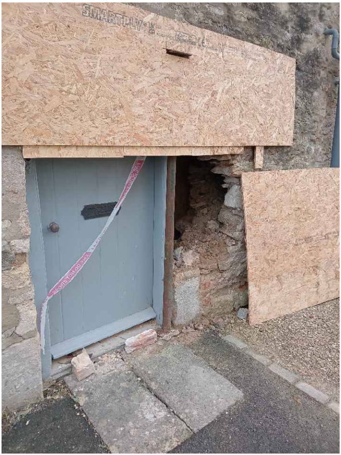
Photo 2: View of the damage caused externally
