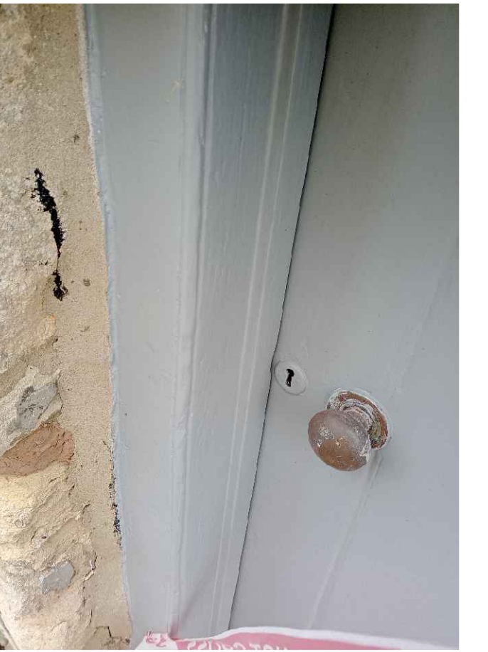
Photo 5: Photo of in tact jamb, to be replicated
