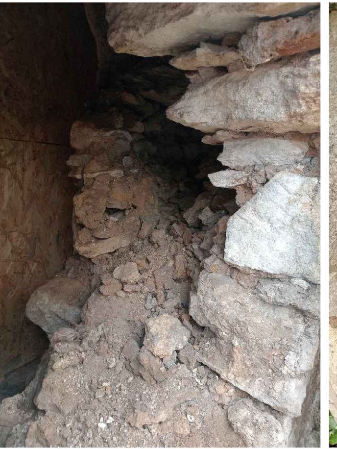
Photo 5: Close up of the damage to masonry
