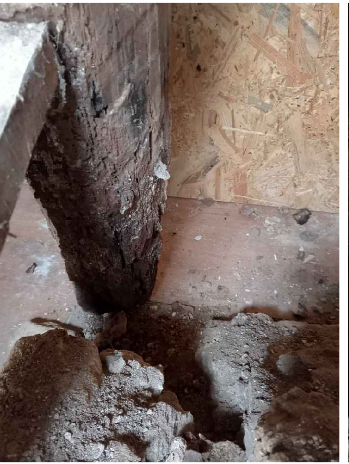
Photo 4: Decay to the dislodged timber post (assumed Elm)
