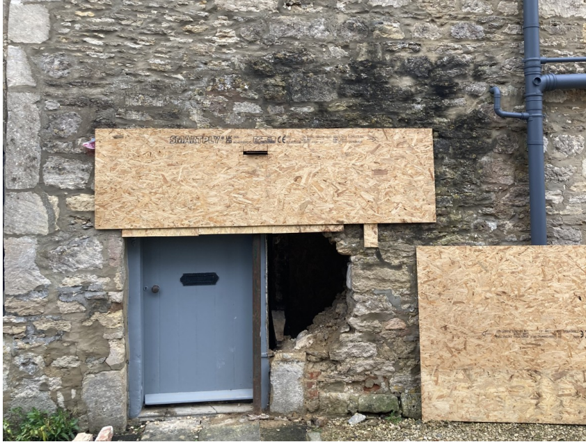
1. Collapsed section of the side wall with visible black mould and staining.
