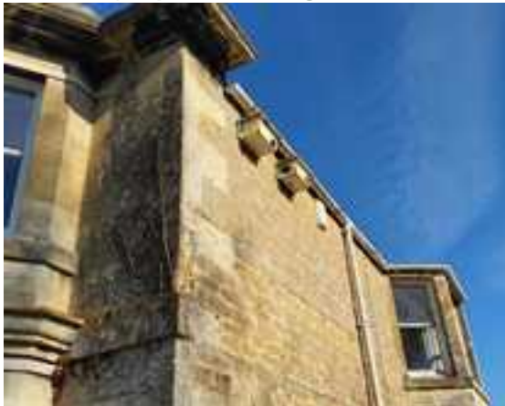
Figure 3: The bird boxes on the east elevation have multiple entrances likely caused by squirrel damage
