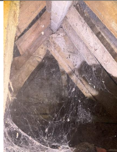
P10 Thick cobwebs in loft
