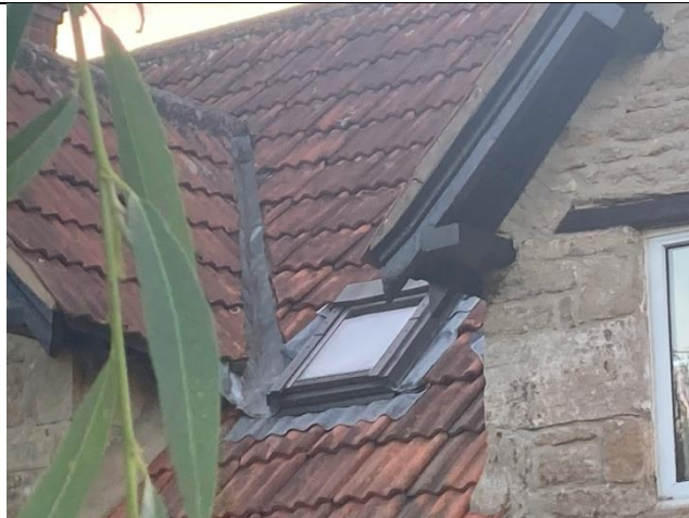
P7 Gaps around dormer windows and roofline
