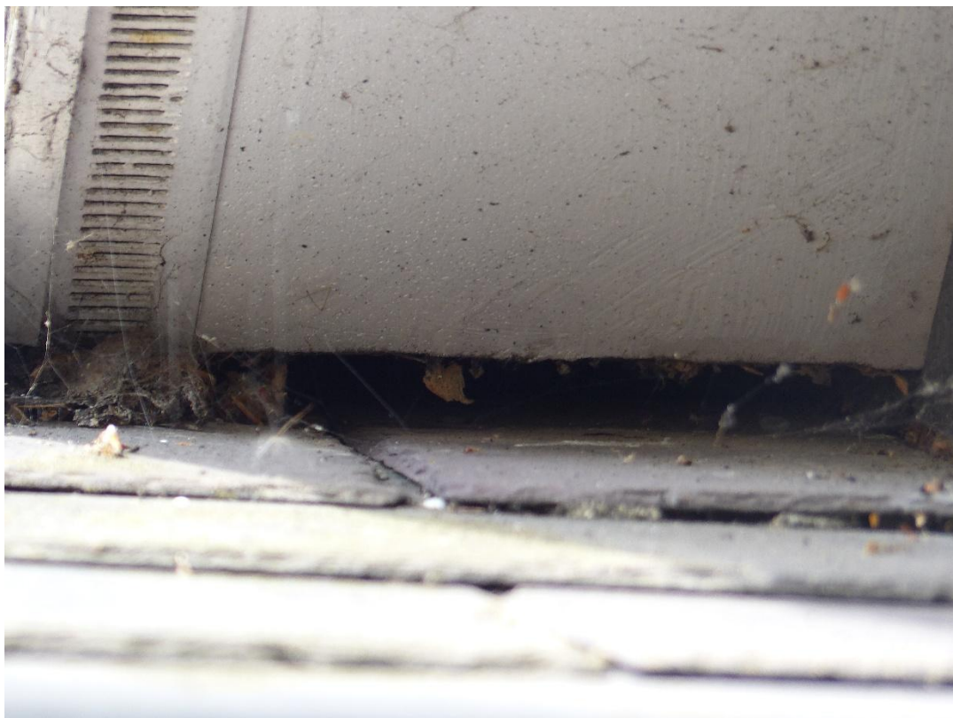
Figure 14 – Gap between slates and dormer soffits, eastern aspect
