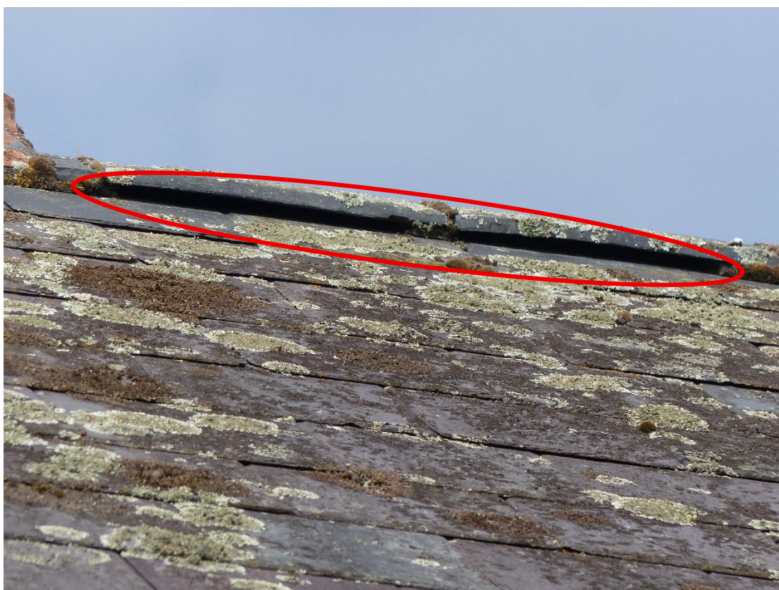
Figure 11 – Gaps below ridge tiles on eastern-facing roof
