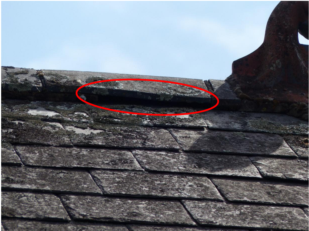
Figure 13 – Gaps below ridge tiles, western aspect
