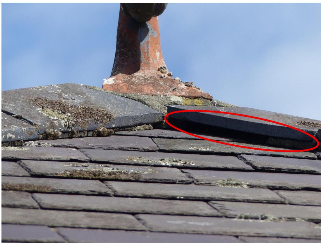
Figure 10 – Missing mortar below ridge tile on southern hipped section of roof
