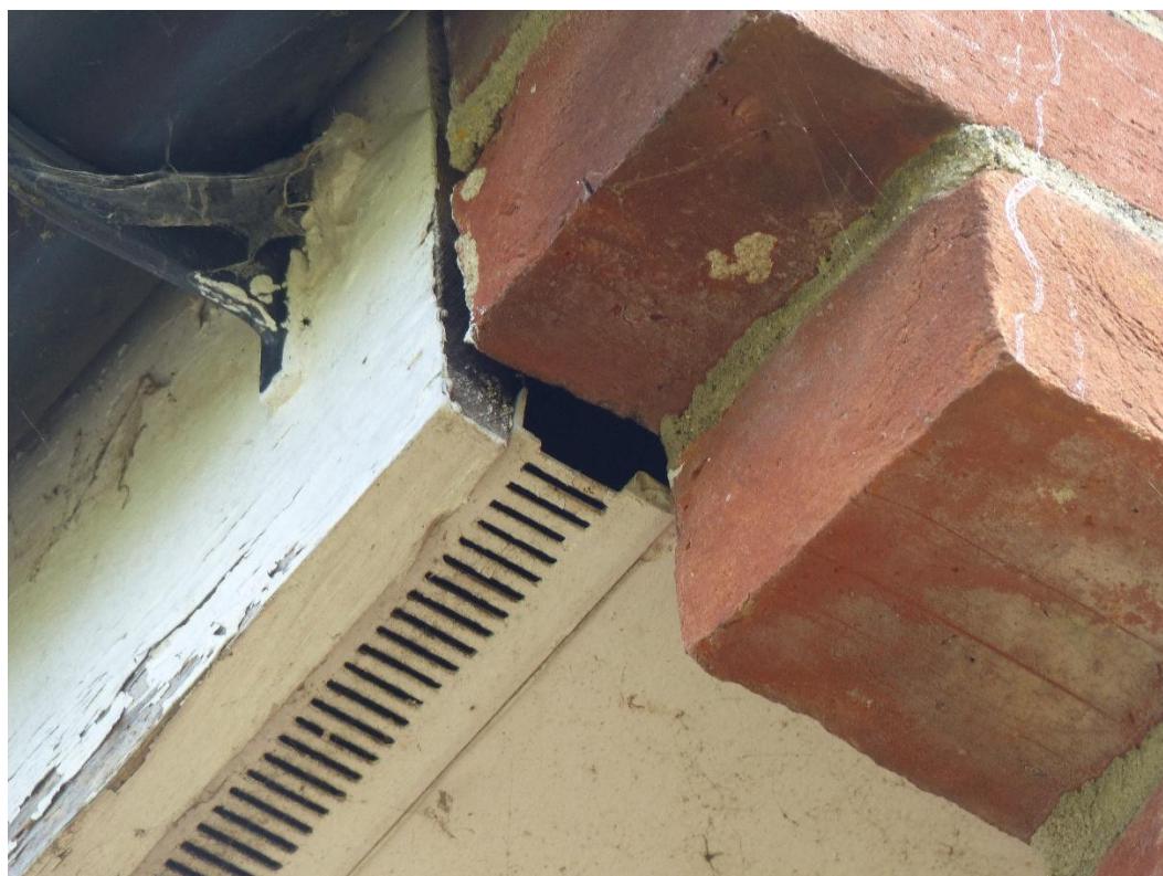
Figure 15 – Gap in soffits (southwestern aspect)
