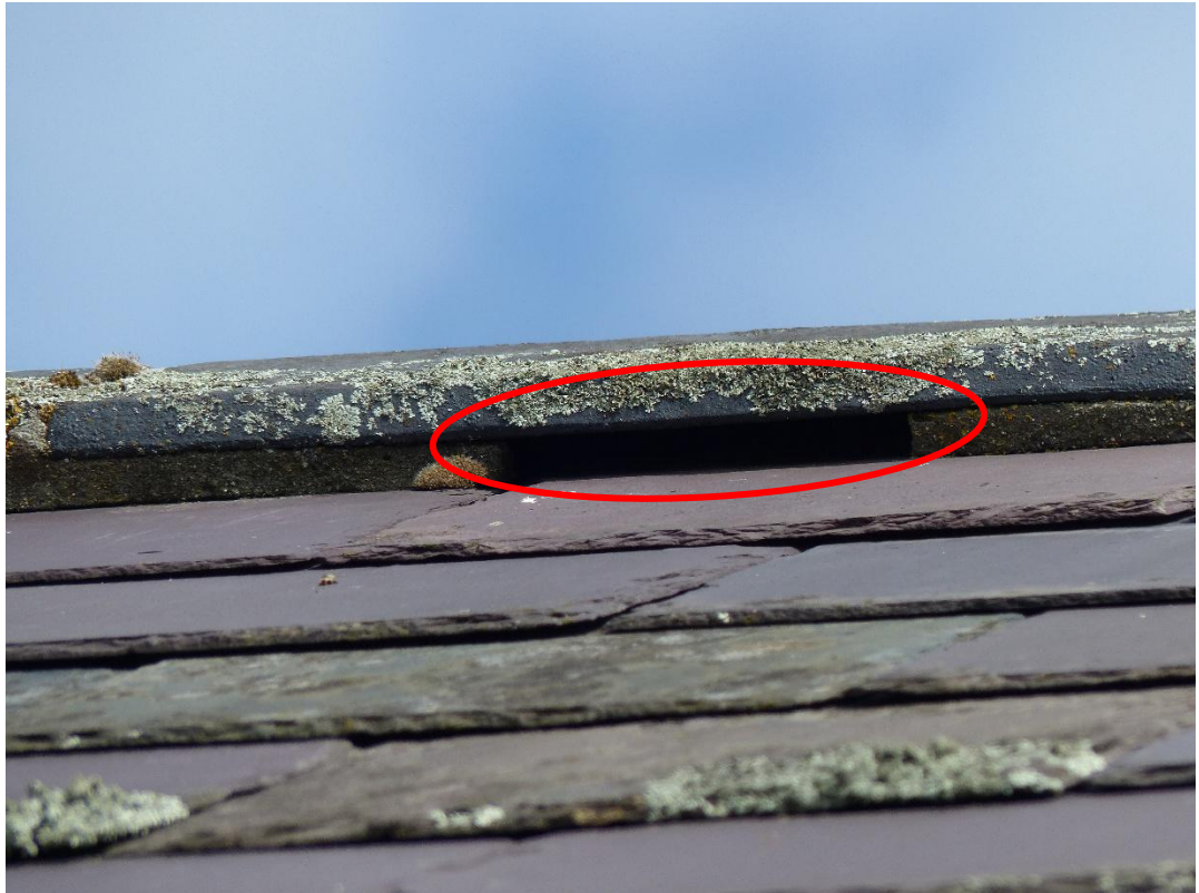
Figure 12 – Missing mortar below ridge tile (southwestern aspect)
