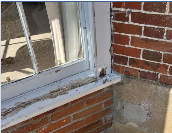
Bay window sash box rot and wall junction
