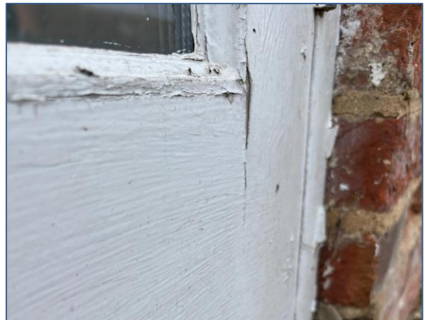
Door bottom rail in poor condition
