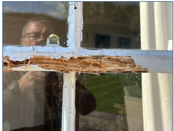
Wet rot to glazing bar
