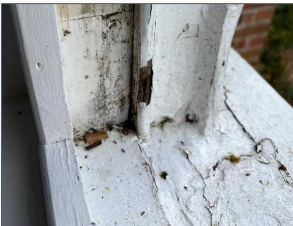
First floor sash box deterioration
