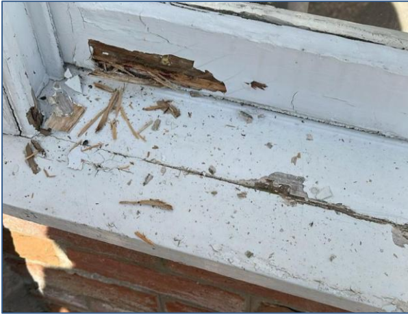
Bay window bottom rail rot
