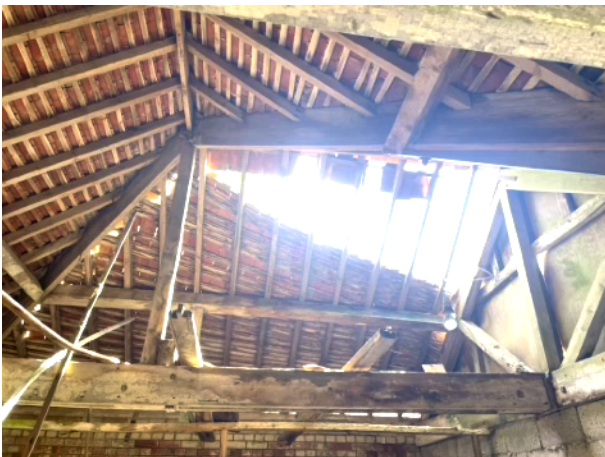
Figure 10. Hole in roof of Barn 1
