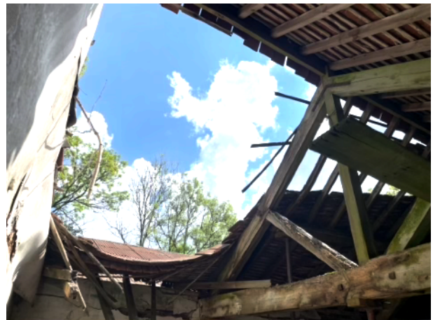
Figure 11. Another large hole in Barn 1 roof
